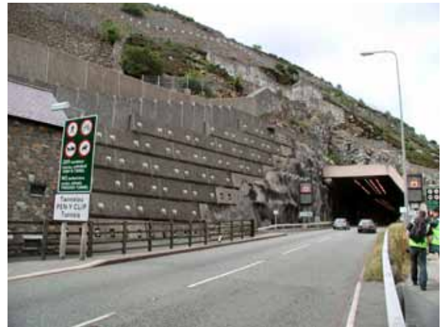
Multiple rockfall protection systems installed near the Pen-Y-Clip tunnel on the A55 North Wales Expressway, United Kingdom. (Photograph: David Giles, University of Portsmouth, United Kingdom)
