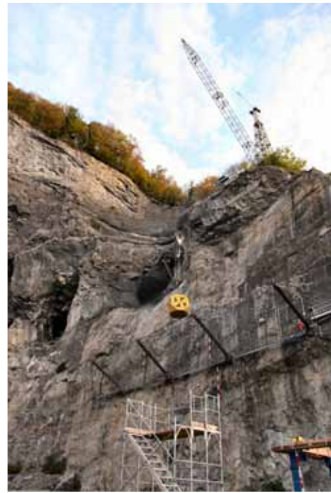
Walenstadt test facility, Switzerland. (Photograph: Geobrugg)
