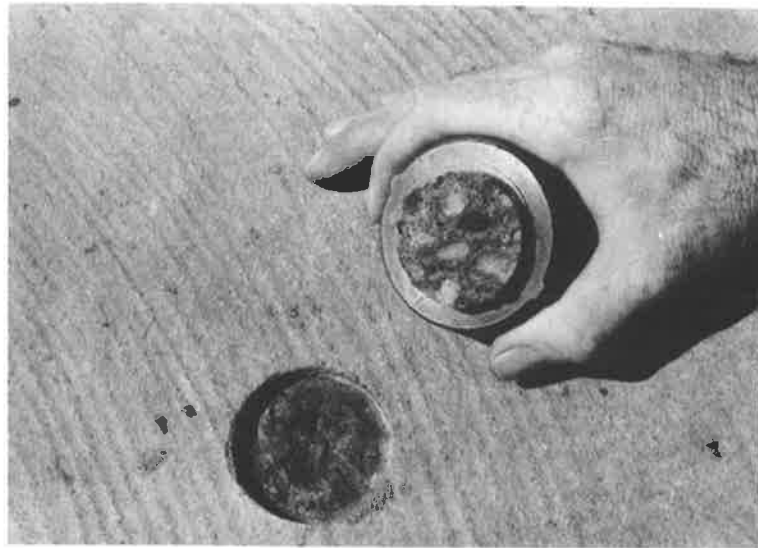
Figure 11. Typical cohesive bond failure in concrete.
