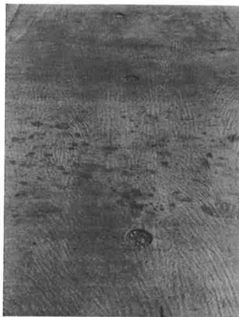
Figure 3. Condition of polyester mortar section after 4 months' service.
