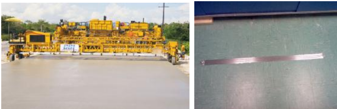
Fig. 5.1 Potential of integration of a novel strip TDR sensor with paving operation
