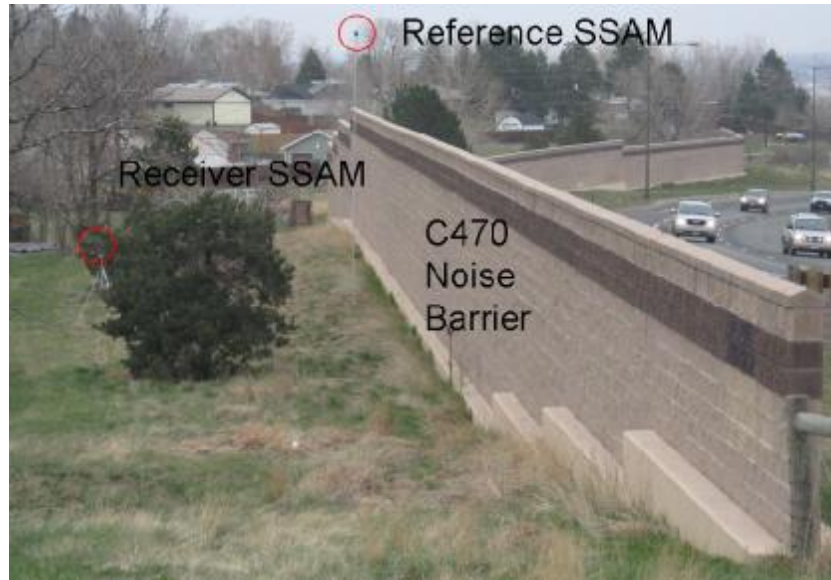
FIGURE 10: After site SSAM configuration. The reference SSAM unit is 1.7 m above the sound barrier. The receiver SSAM unit is 1.5 m the ground.
