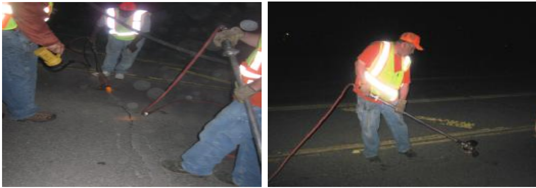
FIGURE 4: NDOR crews using a conventional hot air blaster (left) and the new device (right).
