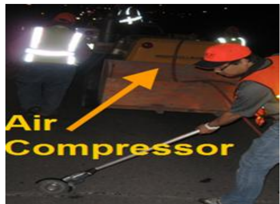
FIGURE 8: NDOR road maintenance air compressor
