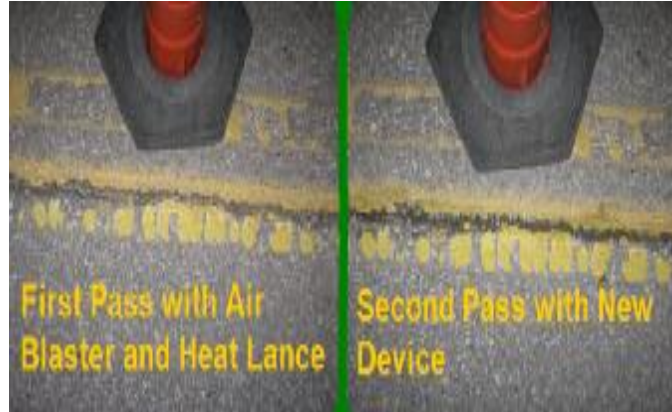
FIGURE 15: A crack after air blasting/heat lance (left) and the same crack after being cleaned by the prototype device (right).
