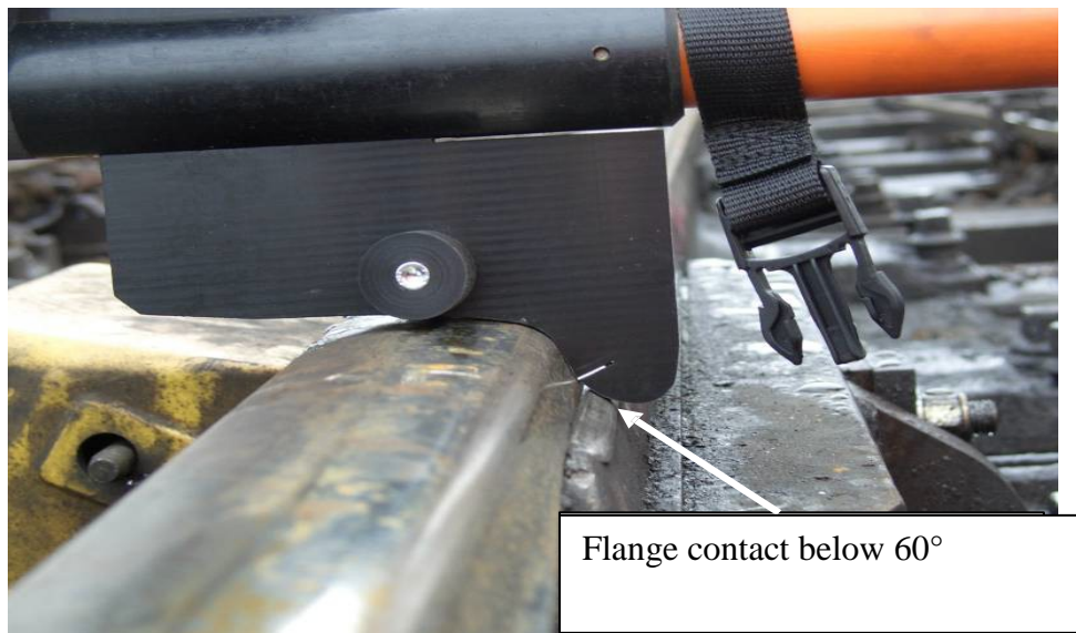
Figure 2: TGP8 Gauge showing switch point contact below the 60° mark – unsafe.
