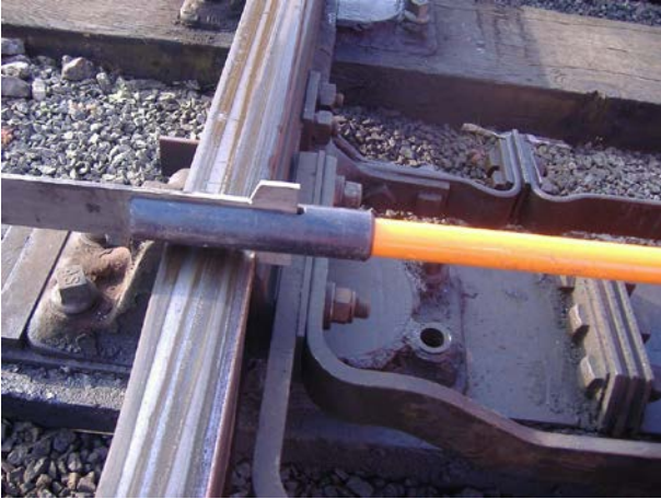
Figure 4B: Switch Gauge 1 used to inspect for stock rail headwear associated with a less worn switch rail.
