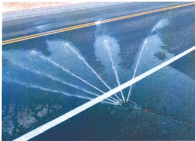
Automated anti-icing spray system for bridge decks
