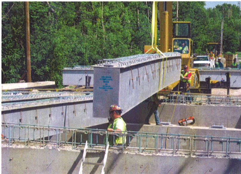
Hybrid Composite Beam (HCB) being installed on High Road Bridge in Lockport Township, Illinois
