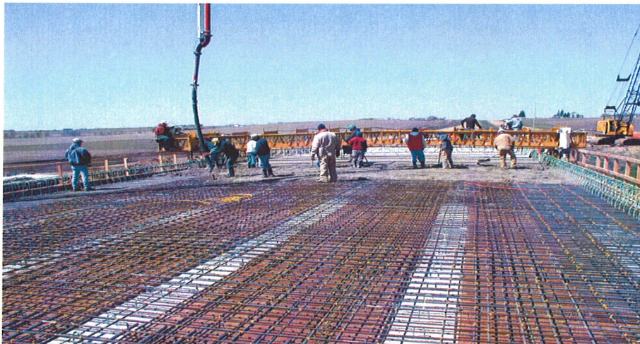
MMFX steel deck reinforcement for US 20 Bridge over South Beaver Creek in Gundy County, Iowa
