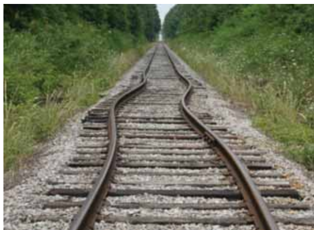
Kinked rail near Fort Campbell, Colorado. Photo courtesy of D.R. Uzarski, Ph.D., P.E., University of Illinois at Urbana-Champaign, Railroad Engineering Program.
