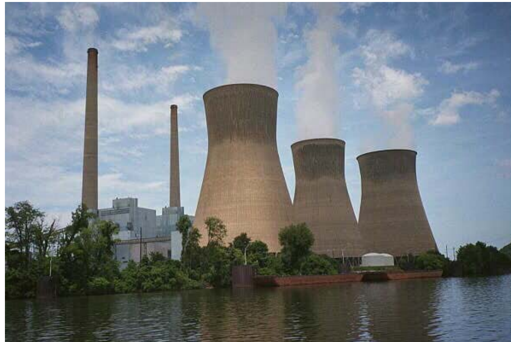
American Electric Power's John C. Amos Plant – Kanawha River Mile 39.2 Photo by Tim Smith, US Army Corps of Engineers
