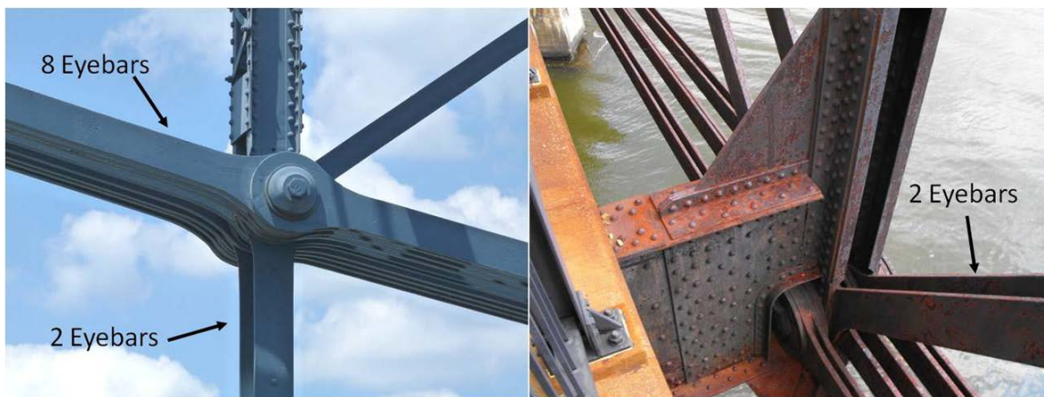
Figure C-2. Examples where failure of one eyebar of the two-eyebar will not result in excessive pin rotation.
