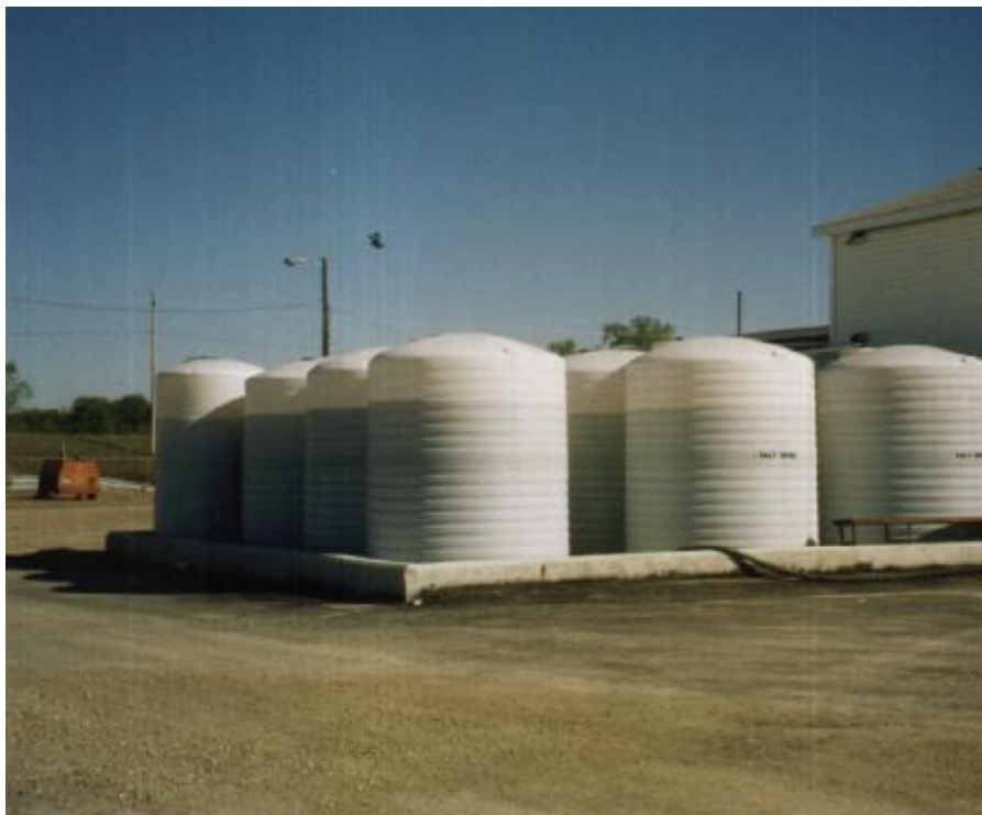
Figure 1. Brine Storage Tanks in Use by the Iowa Department of Transportation.
