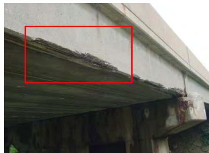
c) prototype girder in situ (photo from PennDOT inspection report dated August 8, 2007).
