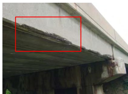
c) prototype girder in situ (photo from PennDOT inspection report dated August 8, 2007).
