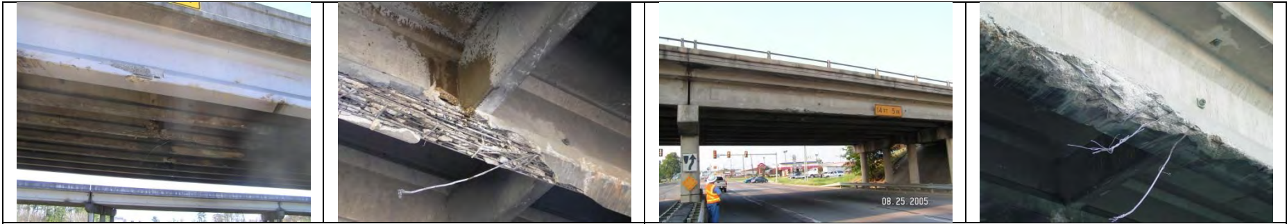
US59 over LP287 (note previous repair material in fig b) AASHTO I-girder; reportedly repaired [Courtesy of the Texas Department of Transportation, © 2007 All rights reserved.]
