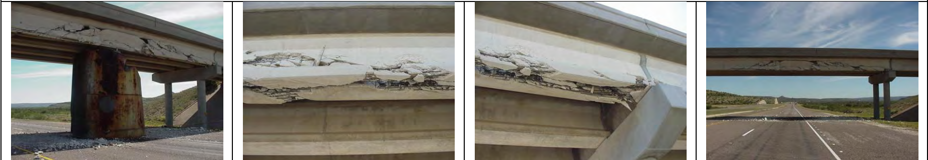
RM215 over IH10, Pecos Co. TX. AASHTO I-girders; reported that only exterior girder was replaced [Courtesy of the Texas Department of Transportation, © 2007 All rights reserved.]
