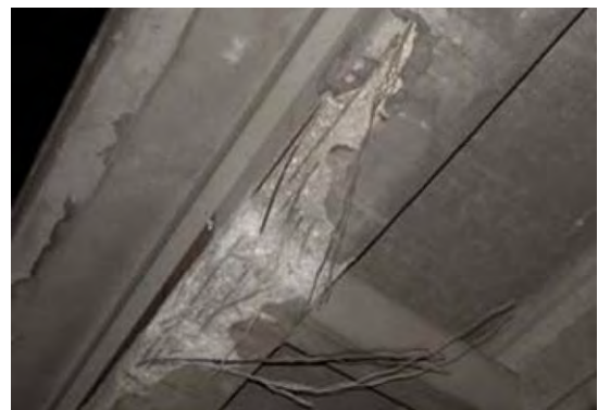
d) damage to exterior girder.
