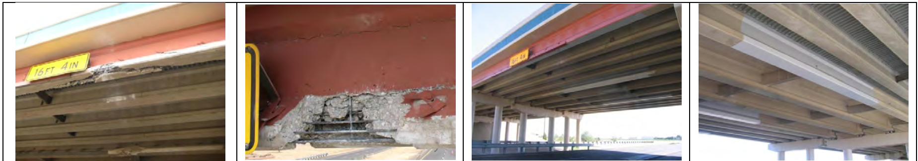
FM 1788 over IH20 AASHTO I-girder [Courtesy of the Texas Department of Transportation, © 2007 All rights reserved.]
