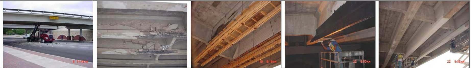
SH6 over SH30 AASHTO I-girder [Courtesy of the Texas Department of Transportation, © 2007 All rights reserved.]
