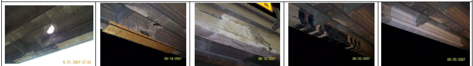
IH-35 at Corinth AASHTO I-girder [Courtesy of the Texas Department of Transportation, © 2007 All rights reserved.]
