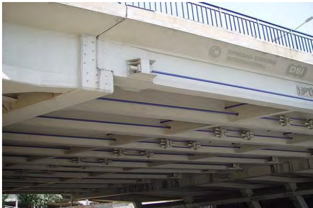
a) PT-steel anchored to girder using steel bolster bolted through girder web (second PT bolster on back of web) [DYWIDAG Systems International]
