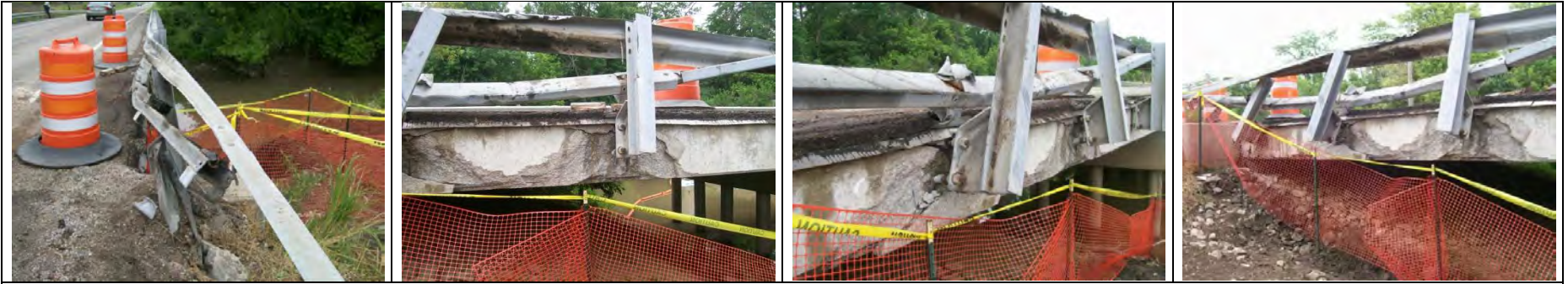
Guardrail impact. reported by source as box beam [ODOT]
