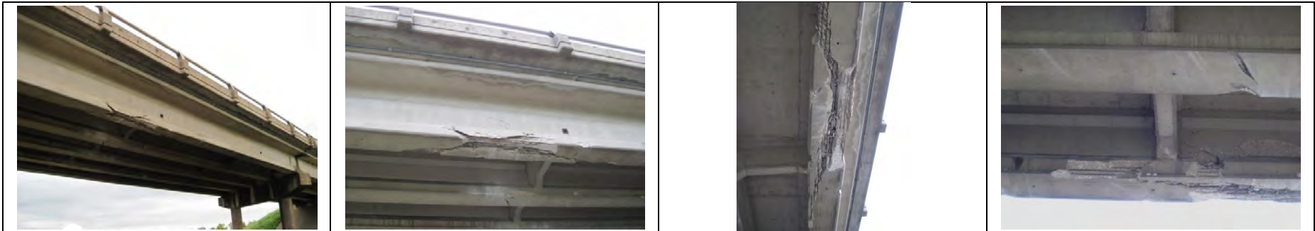
LP301 over IH30 AASHTO I-girder; reportedly repaired [Courtesy of the Texas Department of Transportation, © 2007 All rights reserved.]
