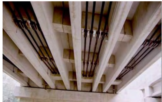
b) PT-CFRP anchored and harped by diaphragms [Mamlouk and Zaniewski Materials for Civil and Construction Engineers 2011]
