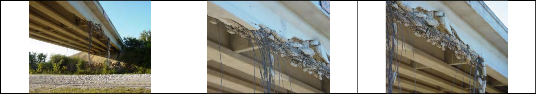
Exterior girder FM479 over Kerr Road, San Antonio TX. AASHTO I-girders; reported that entire bridge was demolished and replaced [Courtesy of the Texas Department of Transportation, © 2007 All rights reserved.]
