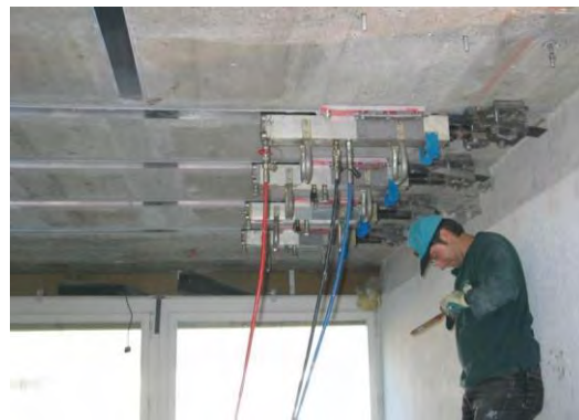
b) live end anchors and jacking system
