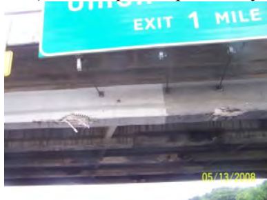
c) 2008 impact to twice-repaired region
