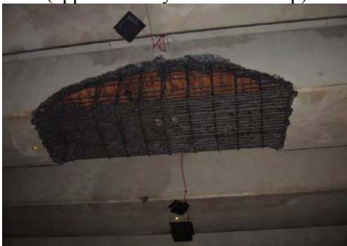
c) damaged region following hydrodemolition
