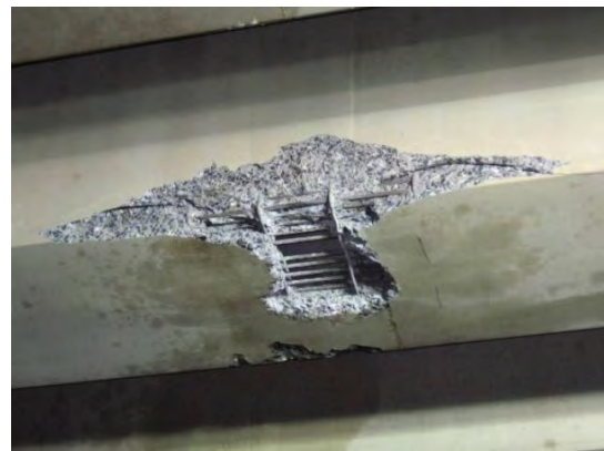
b) damage to fourth interior girder
