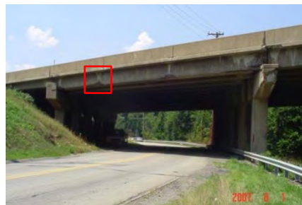
c) prototype girder in situ (photo from PennDOT inspection report dated August 8, 2007).
