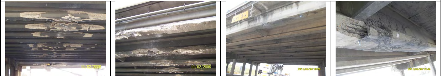
SH 183 at LP12, Dallas TX AASHTO I-girder; reportedly repaired [Courtesy of the Texas Department of Transportation, © 2007 All rights reserved.]
