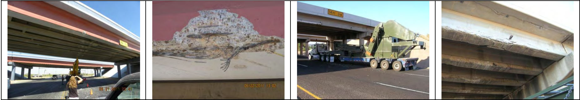
SH 302 at SP450 AASHTO I-girder; reportedly repaired [Courtesy of the Texas Department of Transportation, © 2007 All rights reserved.]
