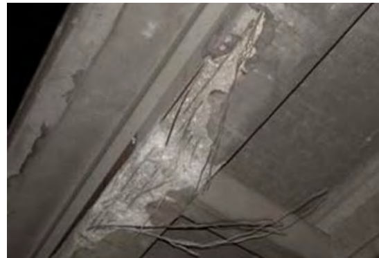
d) damage to exterior girder.
