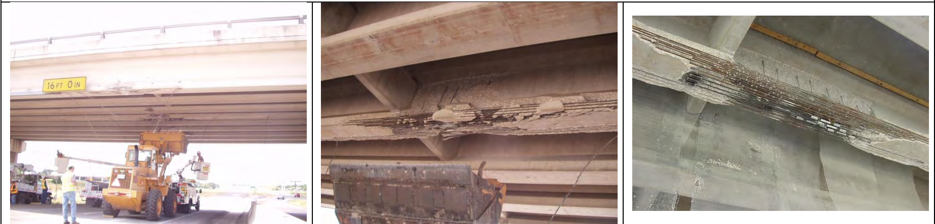
LP363, Temple TX AASHTO I-girder; reportedly repaired [Courtesy of the Texas Department of Transportation, © 2007 All rights reserved.]
