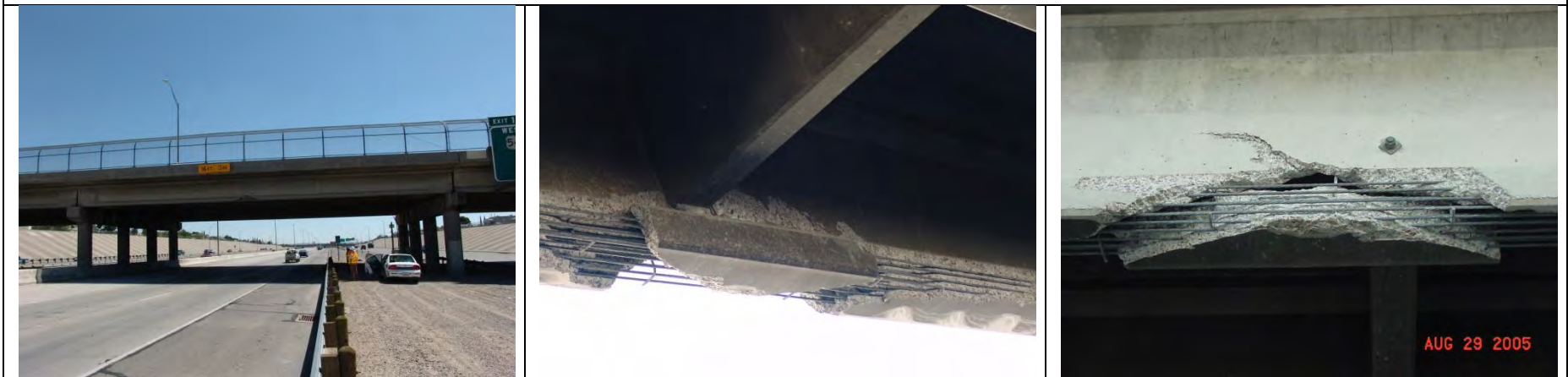
US54 at Altura Ave. AASHTO I-girder; reportedly repaired [Courtesy of the Texas Department of Transportation, © 2007 All rights reserved.]
