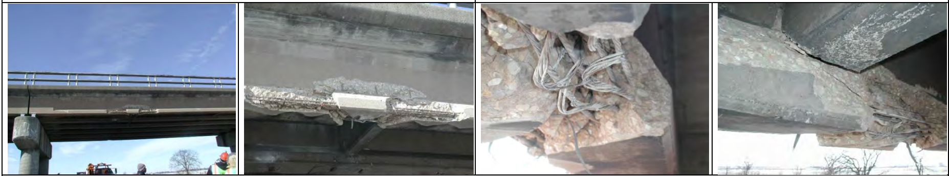
Impact damage to AASHTO I-girder [ILDOT]
