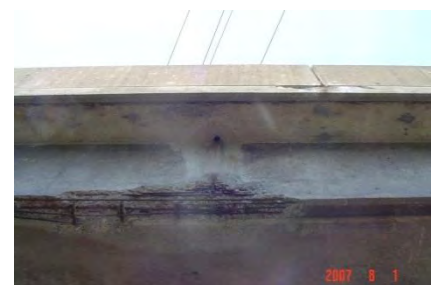
d) impact damage location (boxed location in c).
