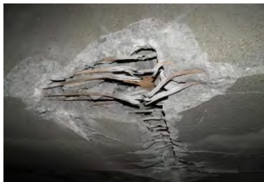
b) Impact damage to fascia beam of McIlvaine Road over I-70. Entire bridge was demolished within 24 hours. [PennDOT]
