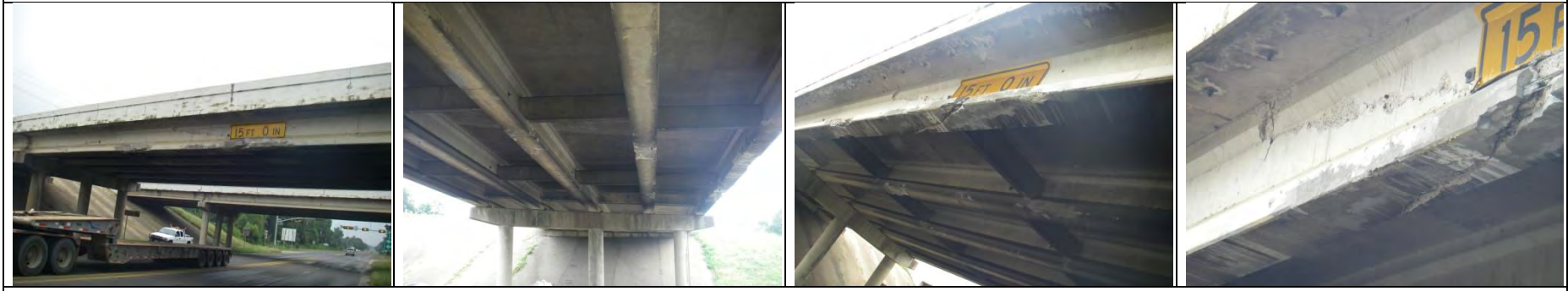
US59 over US79 AASHTO I-girder; reportedly repaired [Courtesy of the Texas Department of Transportation, © 2007 All rights reserved.]
