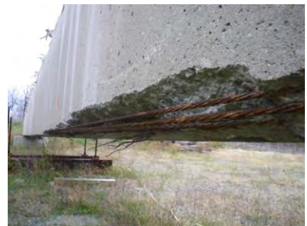
d) impact damage location (boxed location in c).
