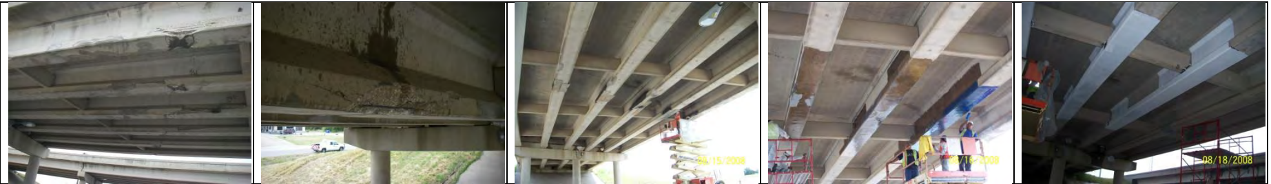
US183 over IH20 AASHTO I-girder [Courtesy of the Texas Department of Transportation, © 2007 All rights reserved.]
