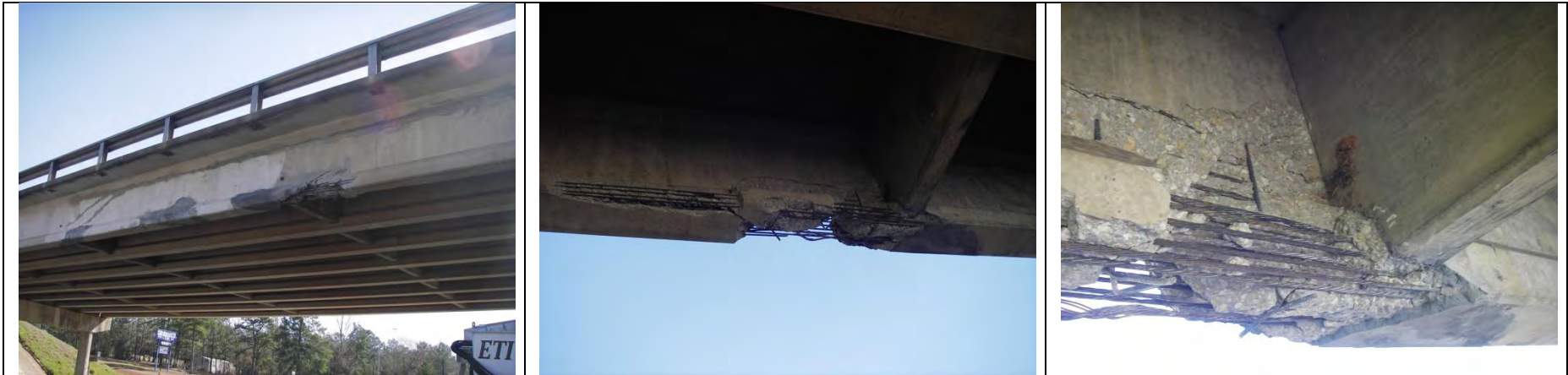
Lufkin TX AASHTO I-girder; reportedly repaired [Courtesy of the Texas Department of Transportation, © 2007 All rights reserved.]
