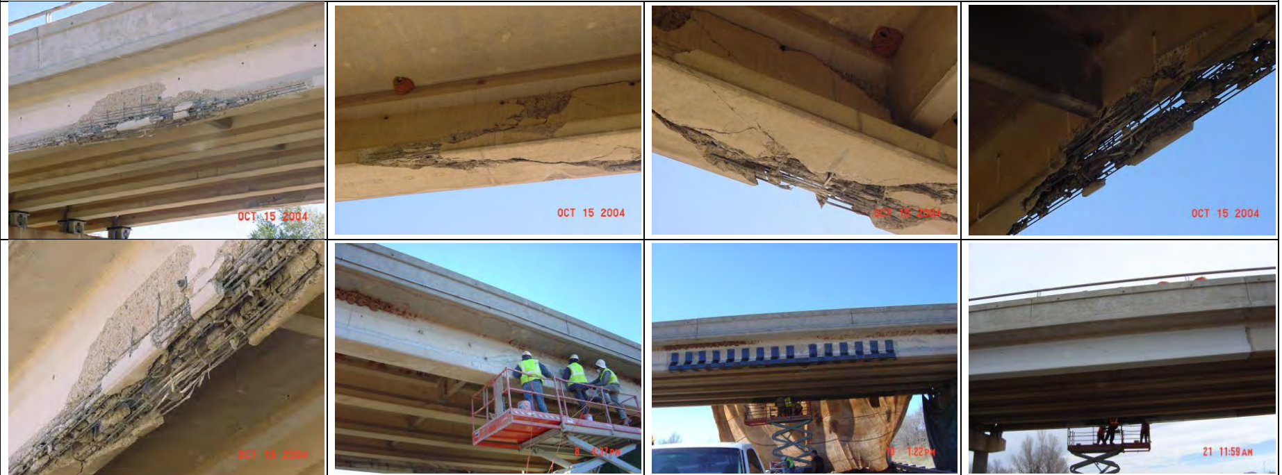
IH40 at Shamrock AASHTO I-girder [Courtesy of the Texas Department of Transportation, © 2007 All rights reserved.]
