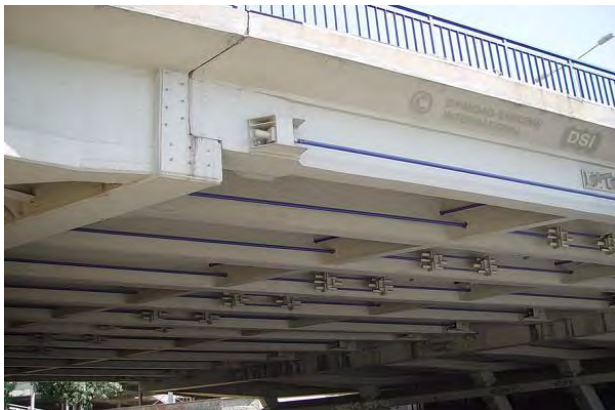
a) PT-steel anchored to girder using steel bolster bolted through girder web (second PT bolster on back of web). [DYWIDAG Systems International]
