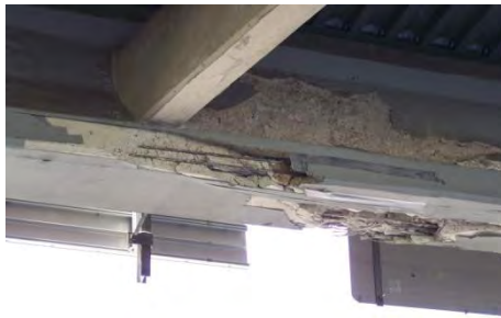
a) 2007 impact to previously repaired region
