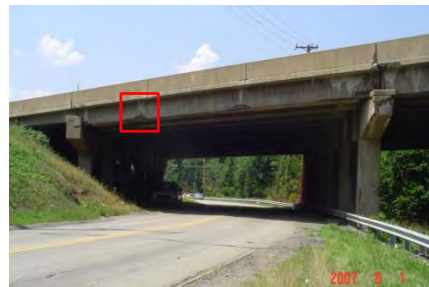
c) prototype girder in situ (photo from PennDOT inspection report dated August 8, 2007).
