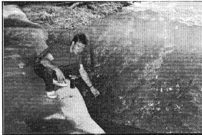
Figure 7.6. Shows grout mass undercut and cantilevered from the adjacent abutment.
