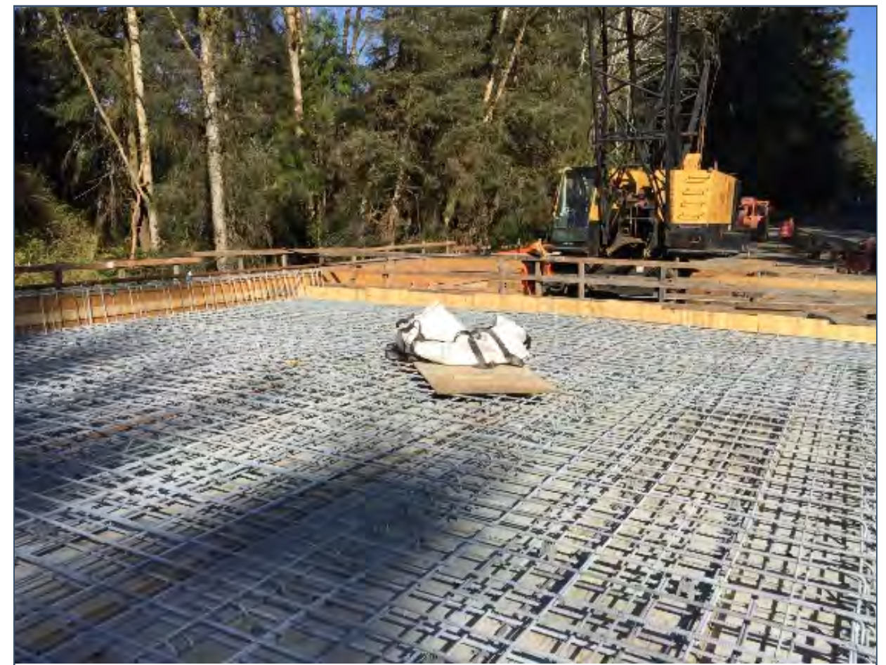
Figure 16. Galvanized reinforcing bars used in a bridge deck exposed to marine salt in the air in Washington
