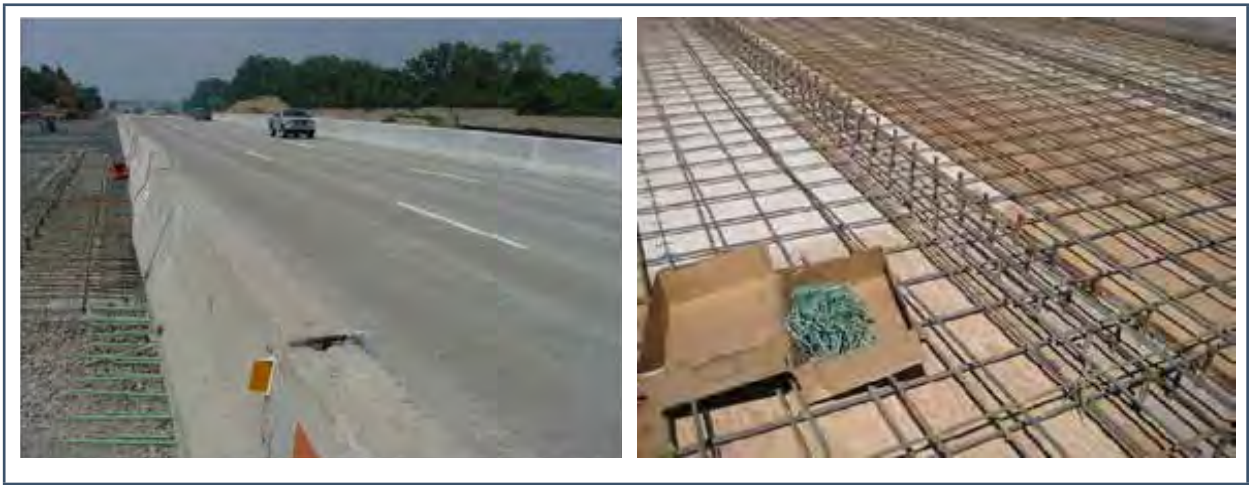
Figure 18. Bridge deck with ASTM A1035 bars built in 2003 in Michigan (left) and in 2008 in Utah (right)
