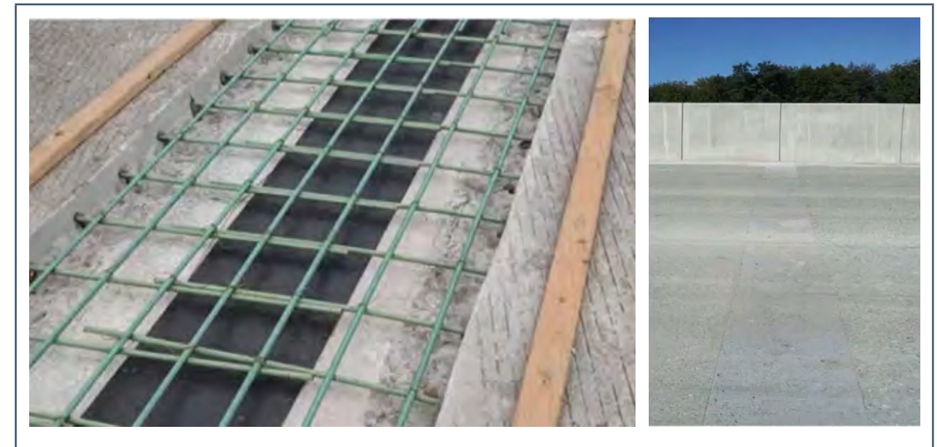
Figure 7. Link slab construction (left), finished link slab (right) from New York State DOT
