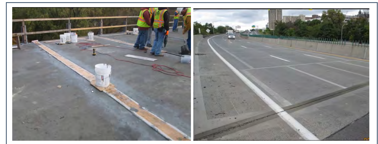
Figure 10. Sealing of precast deck panel forms for UHPC joints (left), finished joints (right) from New York State
