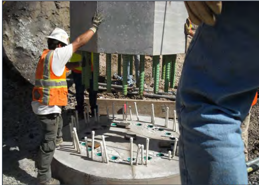
Figure 2.22 Precast column connection to pile shaft with embedded grouted coupler in Utah
