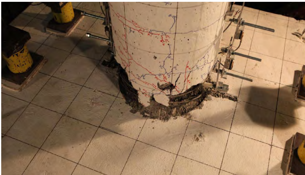
Figure 2.35 Plastic hinge in precast column embedded in CIP footing
