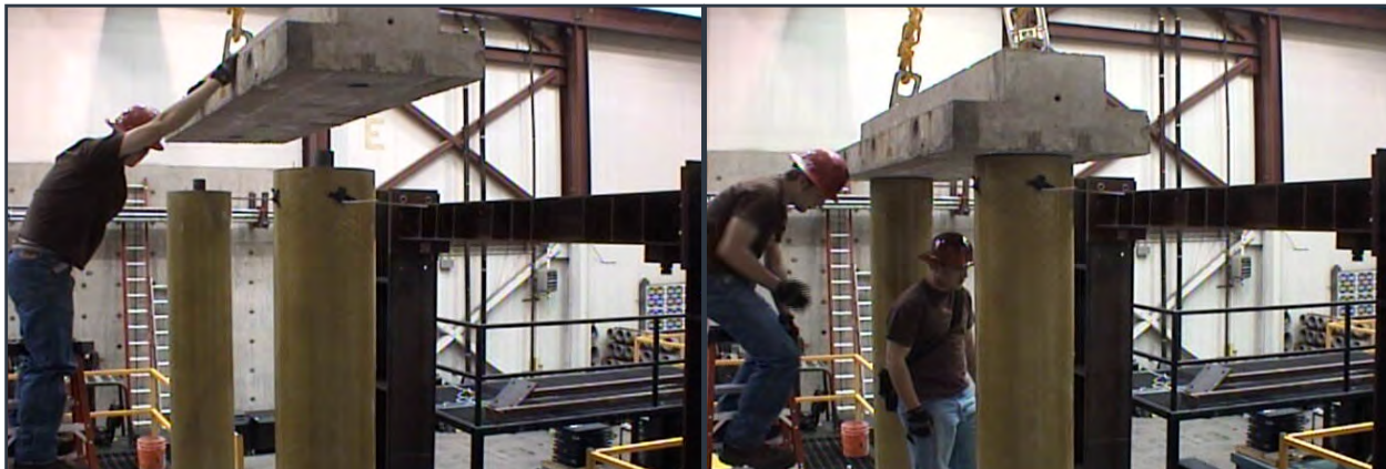
Figure 2.51 Lowering a precast cap beam onto steel pipe pin connections of a concrete-filled FRP tube pier at UNR
