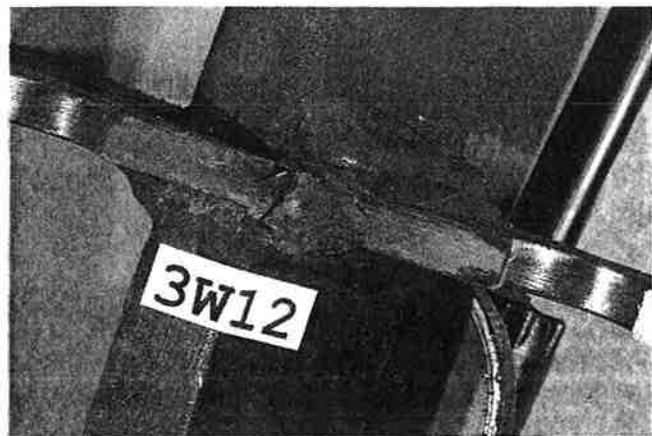
Figure 14. Typical through thickness crack arrested by retrofit holes.
