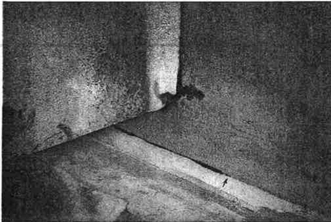
Figure 29. Fatigue cracks at web gap of 1N09.
