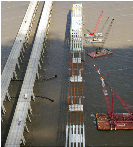
NCHRP research contributed to the accelerated design and construction of the new I-10 Twin Spans Bridge.
