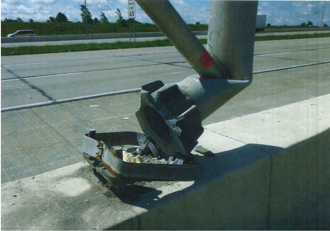
Figure B-13. Overhead Sign Structure Impacted by a Vehicle
