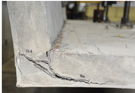
Figure D4. Diagonal cracking of slab
