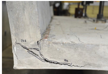
Figure E7. Diagonal joint damage in slab
