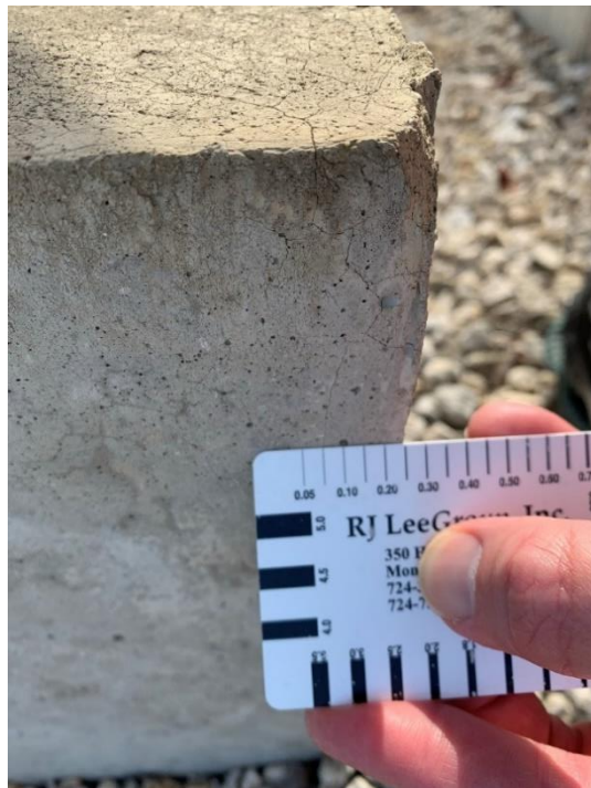
Figure 37. Photo of TxDOT exposure block 64 with hairline cracks on top and extending into the side of the block
