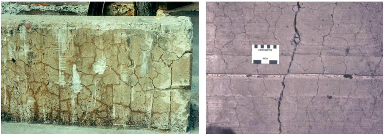
Figure 2. Photograph of ASR in a concrete wall (left) and ACR in a concrete sidewalk (right)
