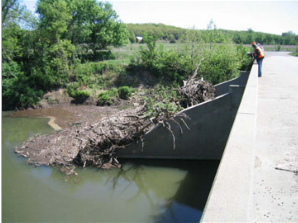
Figure 3.7. Evidence of loss of trees and slope failure on left bank.
