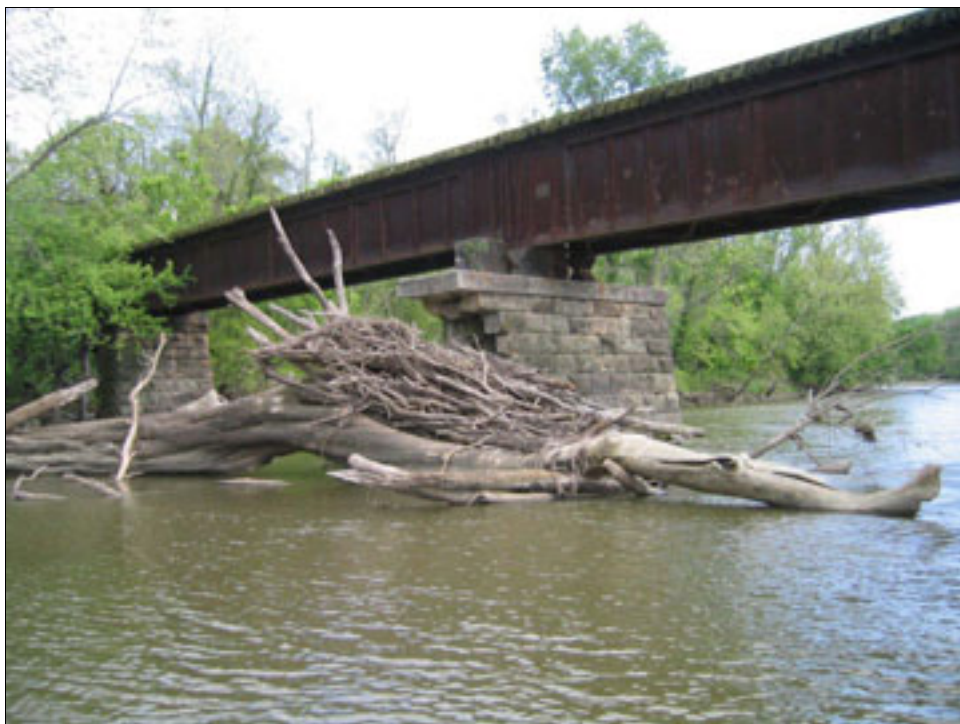
Figure 2.4. Debris at Railroad Bridge pier.
