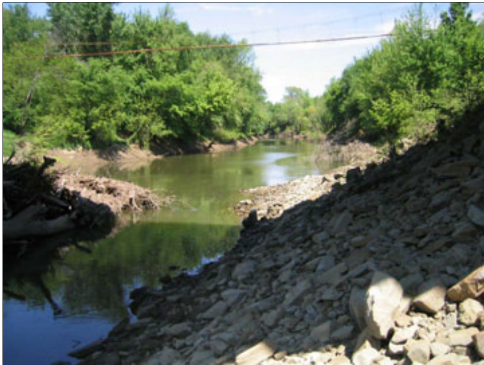
Figure 4.3. Looking upstream from below the bridge deck. Note the riprap on the banks and the trees leaning into the channel.
