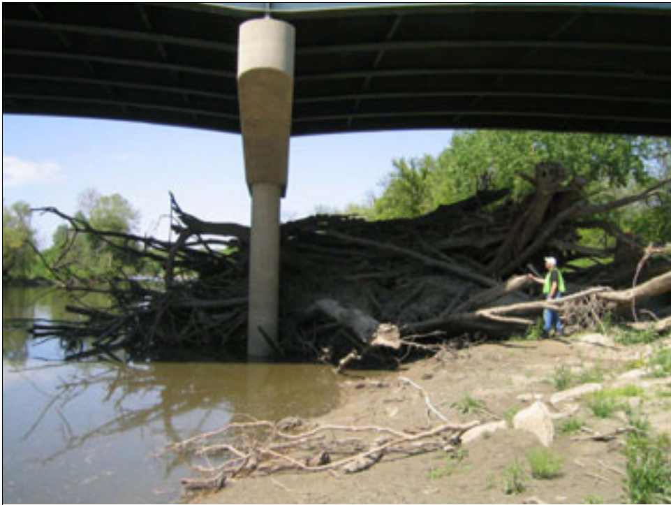
Figure 5.4. Looking upstream at debris pile.
