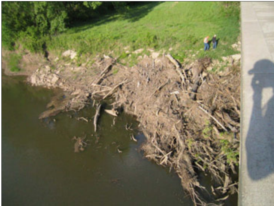
Figure 5.8. View of debris pile from bridge deck.
