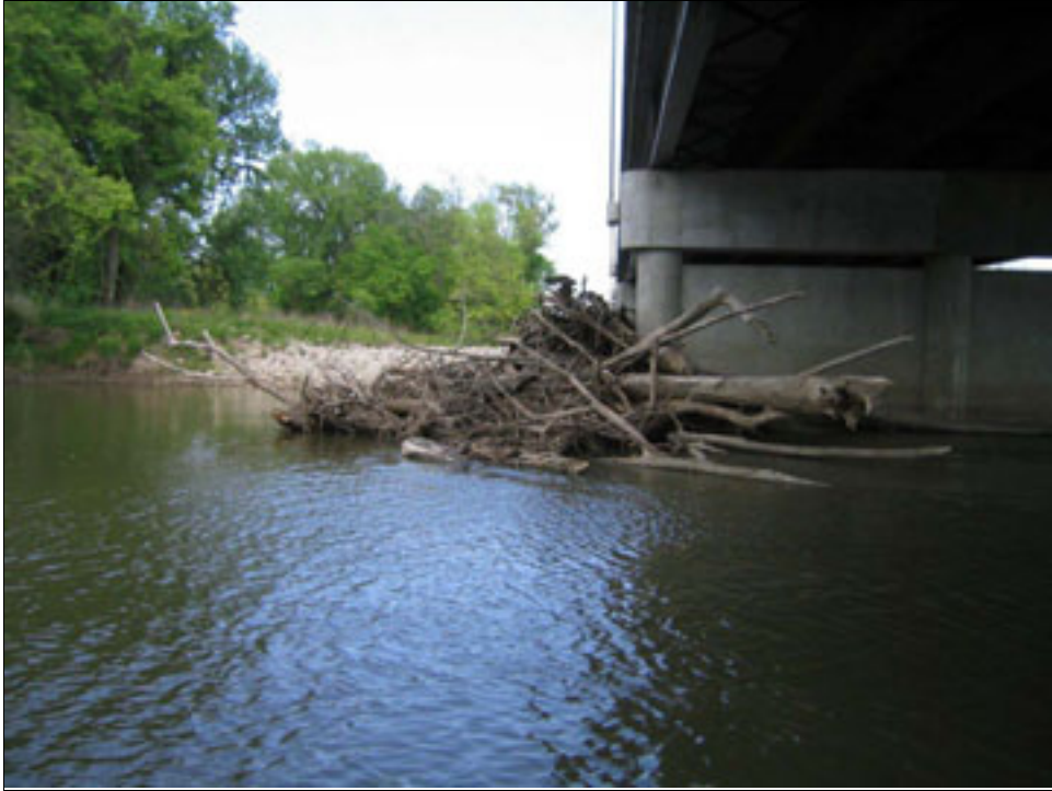
Figure 1.3. Debris buildup at Pier #3.
