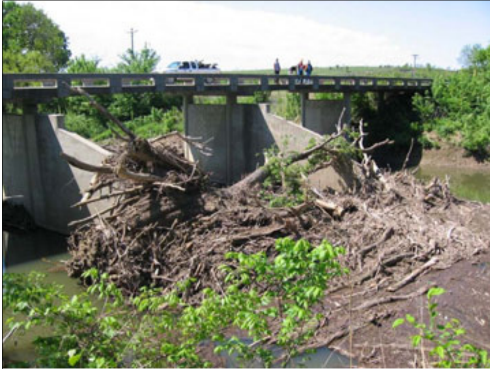
Figure 3.3. Two piers in channel with heavy debris.
