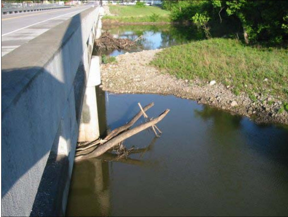
Figure 1.5. Debris at Pier #2. Note the island between Piers #2 and #3.
