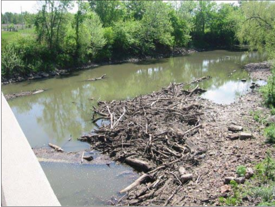
Figure 3.5. Debris removed from piers the previous year and placed downstream of bridge.
