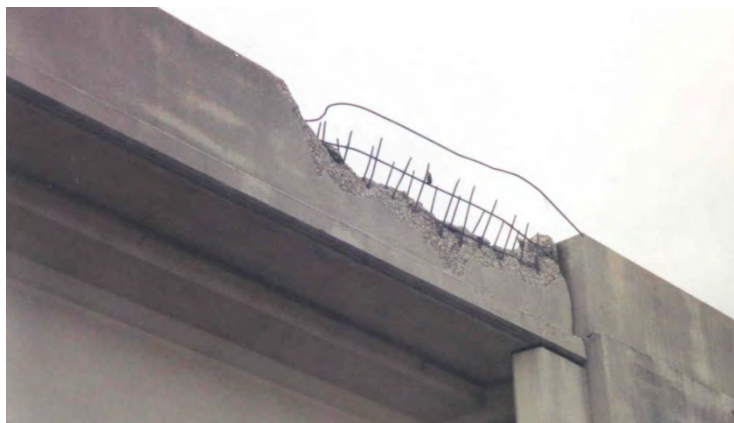
Figure 29. Damage to a 32” concrete bridge railing in a crash with a single unit truck in Florida. [Alberson04]
