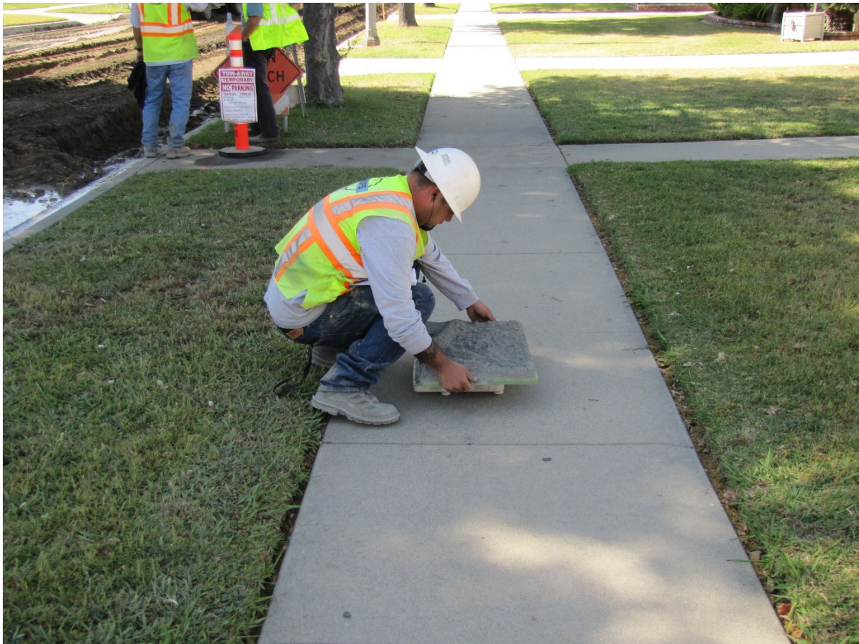
Figure 16 Measuring application rate of active filler using a pan test. (courtesy ARRA)
