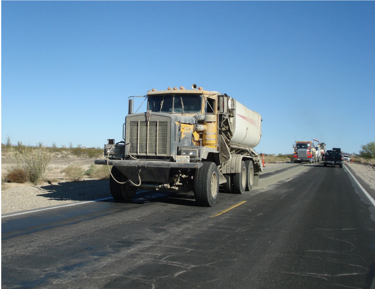
Figure 10 Applying active filler (cement) ahead of a multi-unit CIR train. (courtesy ARRA)
