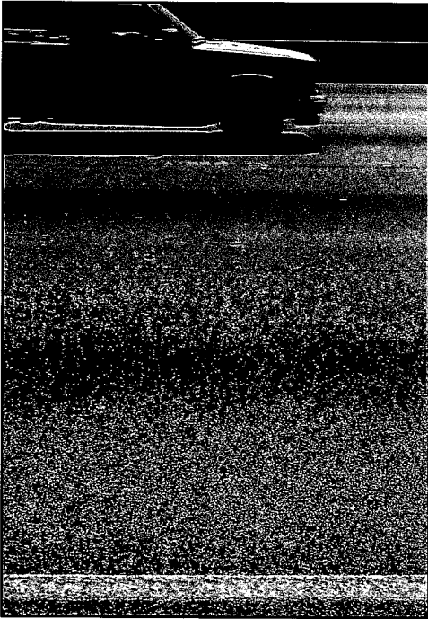
FIGURE 19 ACP 6. Low Severity Transverse Cracking
