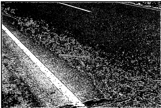
FIGURE 6 ACP 1. High Severity Fatigue Cracking
