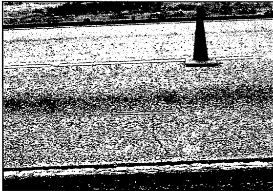
FIGURE 98 CRCP 3. Low Severity Transverse Cracking
