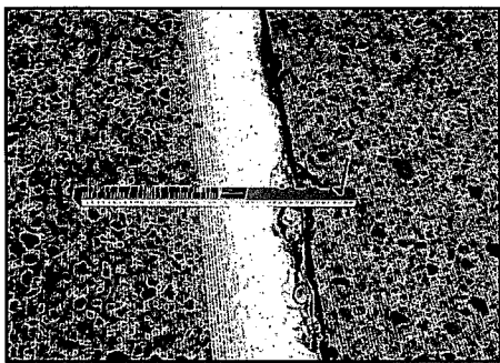
FIGURE 64 JCP 6. Low Severity Spalling of Longitudinal Joint
