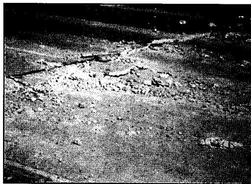
FIGURE 107 CRCP 7. A Blowup
