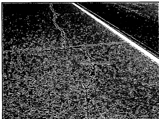
FIGURE 57 JCP 3. High Severity Longitudinal Cracking
