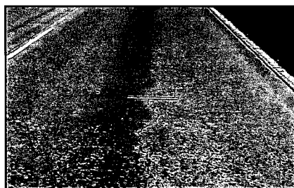
FIGURE 94 CRCP 2. Low Severity Longitudinal Cracking
