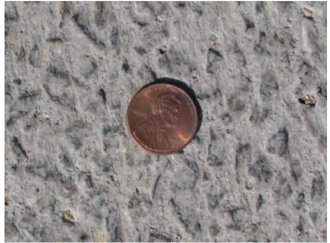
Figure 2: Close-up of a finished exposed aggregate concrete texture that was constructed in Germany
