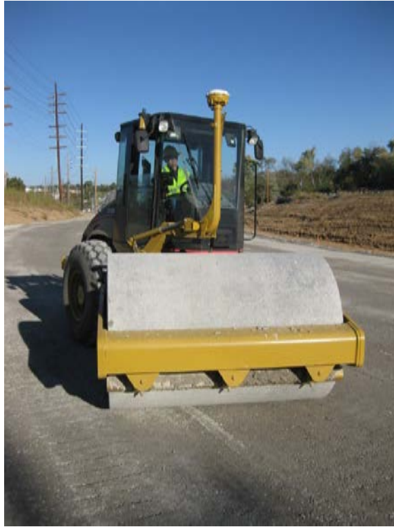
Figure 9: IC roller on Test Area #2 on north end temporary detour road on aggregate base
