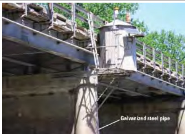
Figure 3: Installed conduit and existing streamgage shelter at structure L-524 site
