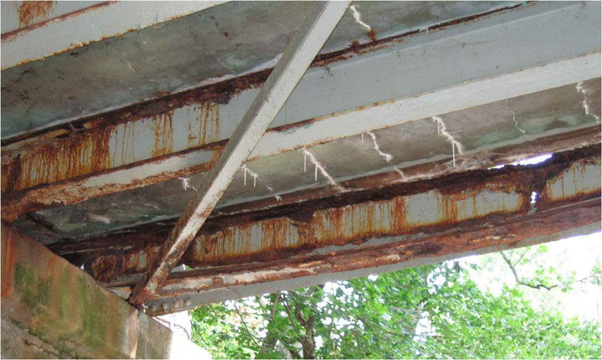
Figure 2: Original stringers, lateral bracing and concrete deck showing sin
