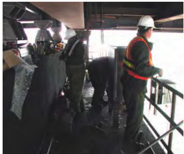
Figure 7: Wiring of river channel-bed monitors
