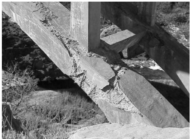
Figure 2: Spalling concrete and exposed steel before renovation
