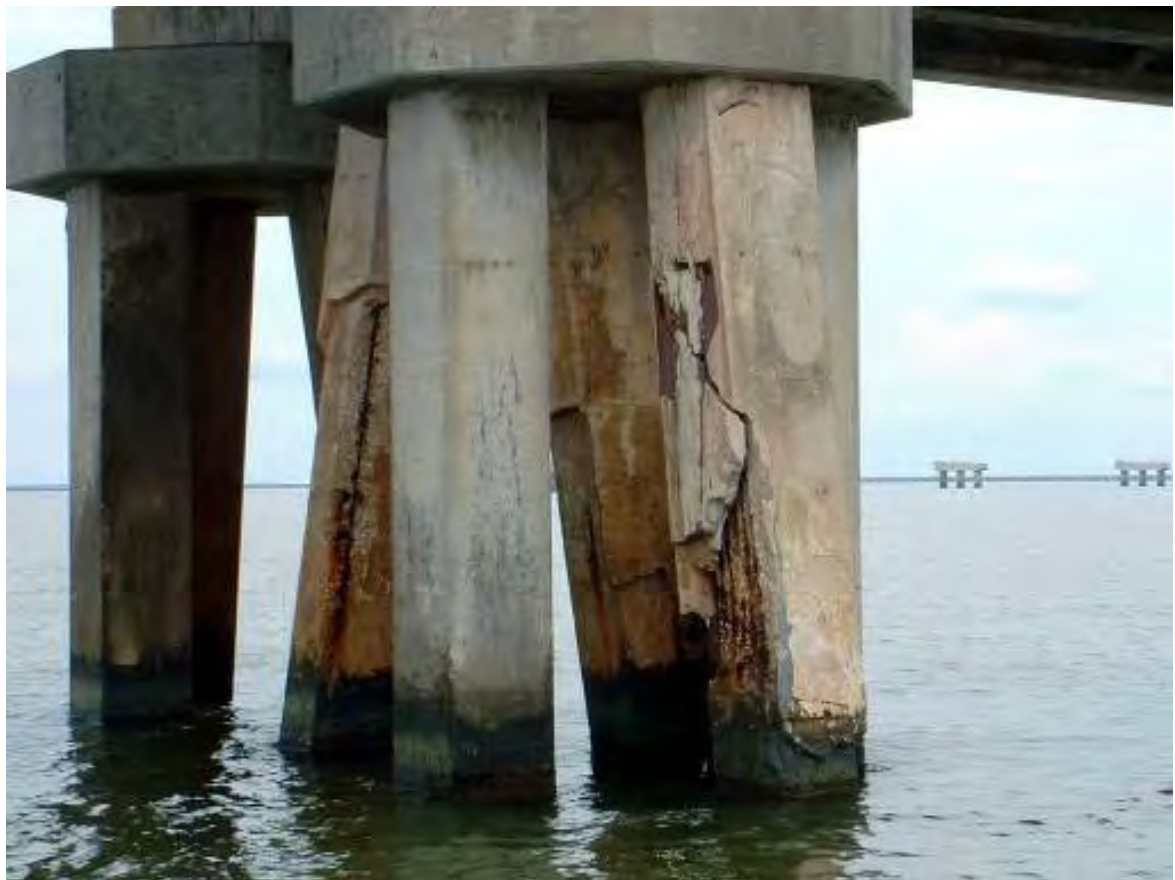
Figure 1: Condition of existing concrete piles at the Key Royale Bridge site before rehabilitation
