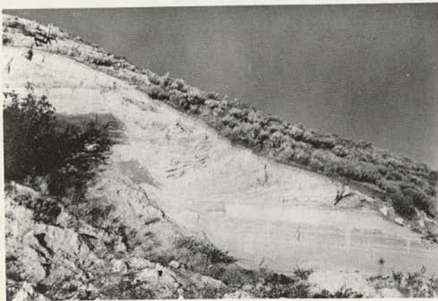
Figure 2.8. Slump in bedded deposits similar to those shown in Figure 2.7 (note that surface of rupture follows horizontal bedding plane for part of its length) (2.182).
