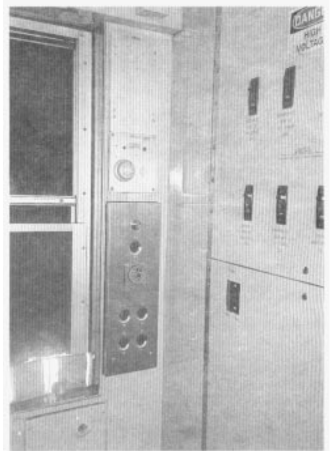
Figure 61. MTA-NYCT door control panel.
