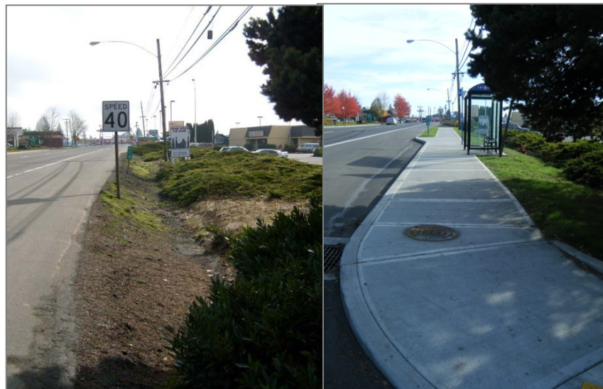
TriMet's Bus Stop Improvements along Tualatin Valley Highway: "Before" and "After" Stops (Photos courtesy of TriMet)
