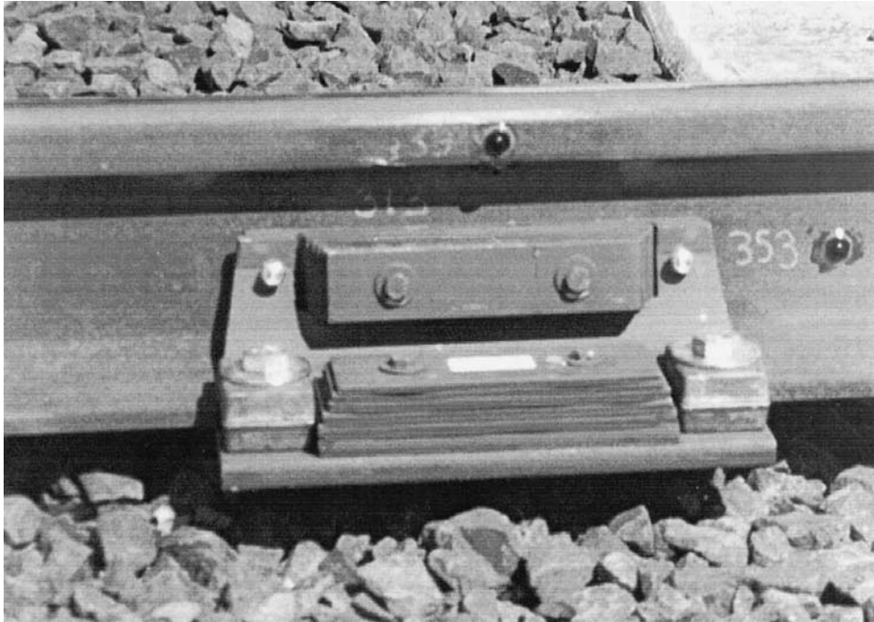
Figure 3. Rail vibration absorber attached to 115 lb/yd RE rail at the Portland Tri-Met ballast-and-concrete-tie track.
