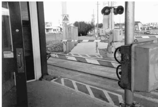
Figure 2-15. Pedestrian automatic gate installation at an LRT station. (Edmonton, Alberta, 129th Ave. crossing.)
