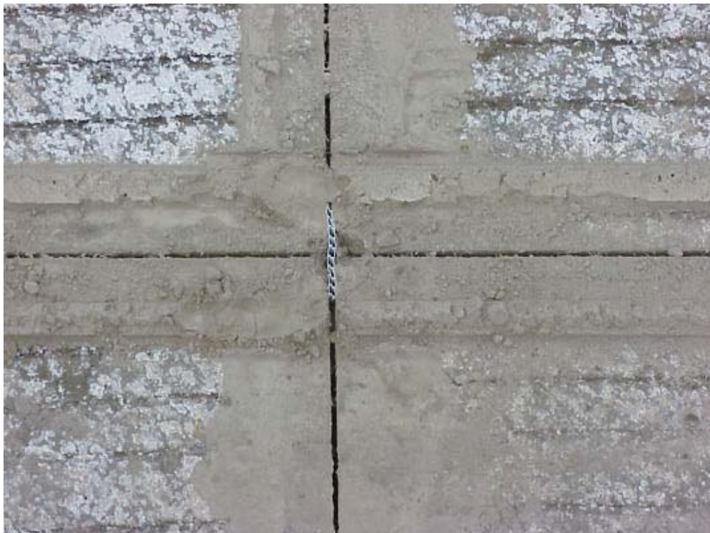
Figure 15 – Plastic spacers are used at the cross cuts to achieve a clean cut
