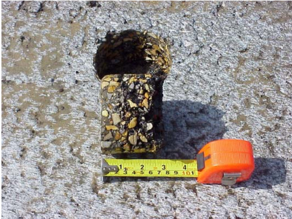
Figure 32 – Entire mat did not get saturated in some areas (1” capping of grout)
