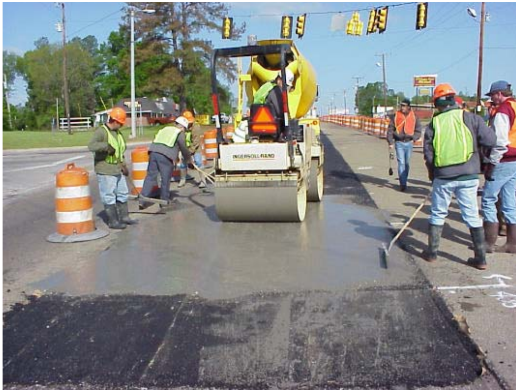
Figure 26 – Using a 3 ton roller in vibratory mode, the grout is forced to penetrate the entire thickness of the 2" open graded asphalt mat
