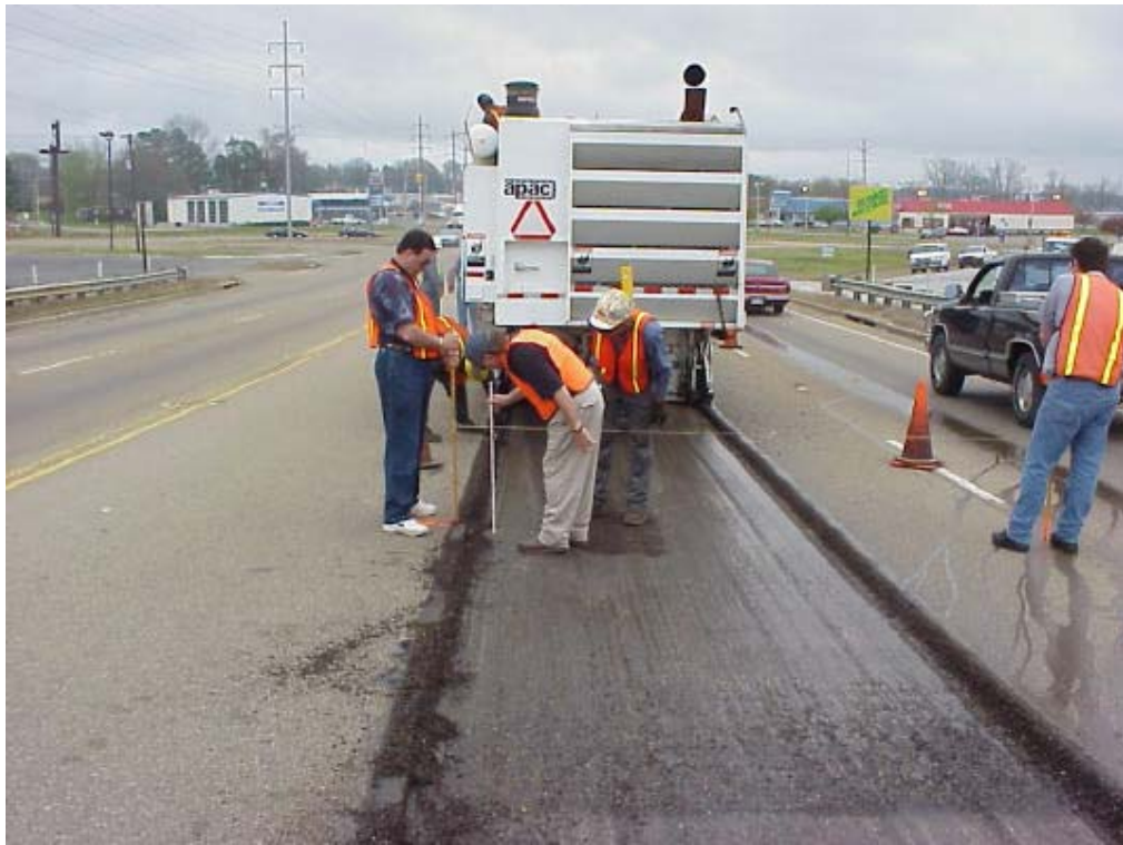
Figure 10 – Milling of the existing asphalt prior to construction of each test section
