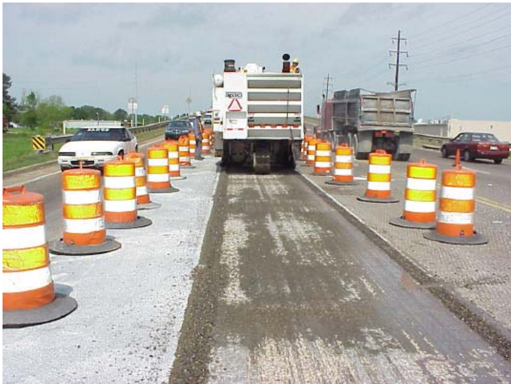
Figure 33 – Milling up of 75' x 12' area that failed to achieve full grout penetration
