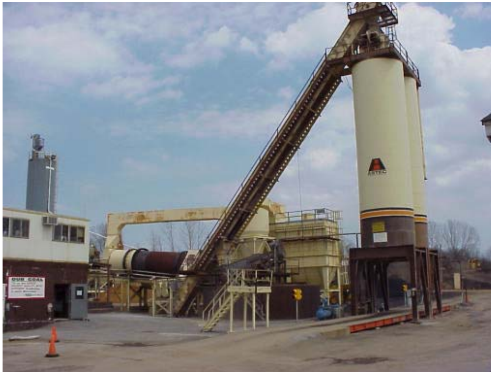
Figure 16 – APAC Corinth “drum” plant which produced both the PG 67-22 open graded mix for the Resin Modified Pavement and the PG 82-22 dense graded mix
