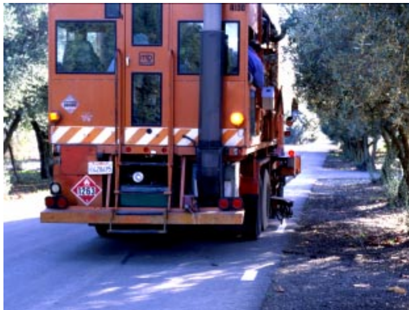
Figure 18. Striping vehicle conducting a test of the longitudinal accuracy of dash line length.
