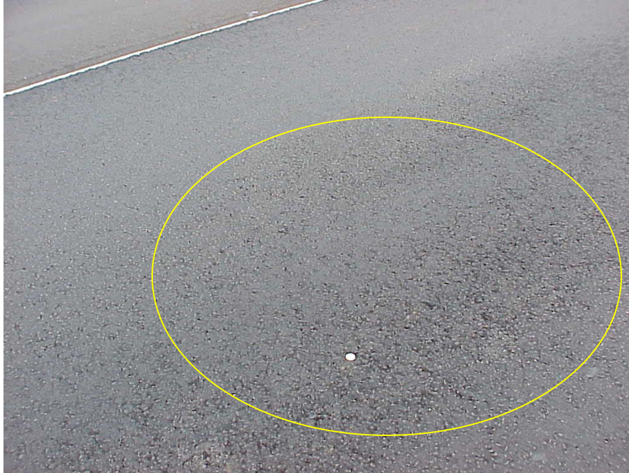
Virgin, Silo, 1.5" Lift Thickness – Open Texture in Compacted Mat Corresponding to Cold Spot
