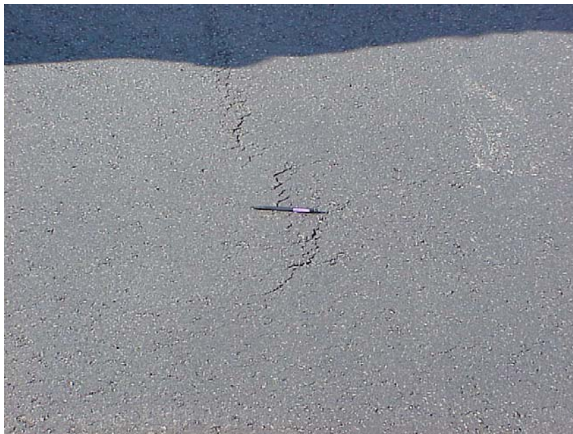
2.0-inch Virgin, No Silo – Cold Rolling Cracks
