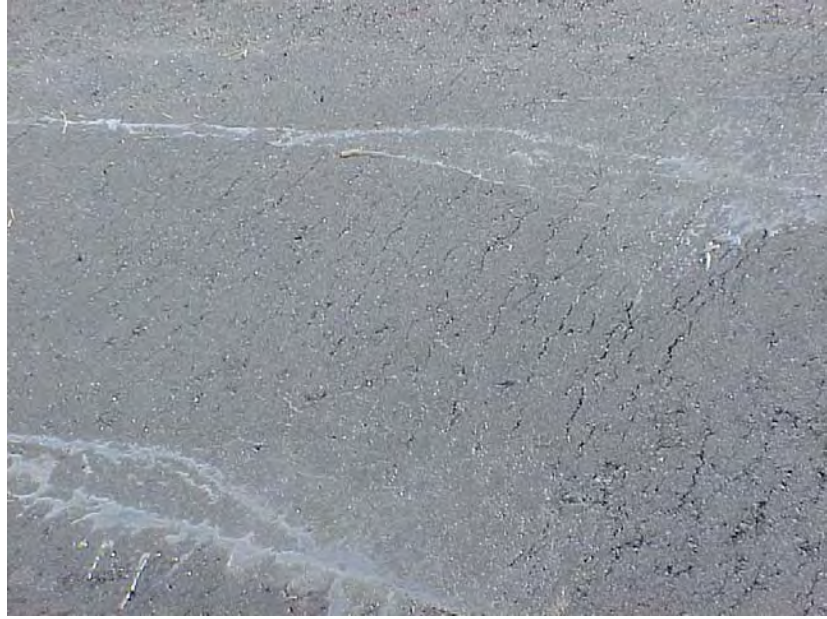
1.5-inch 20% RAP, Silo, Material Transfer Device Used – Cold Rolling Cracks
