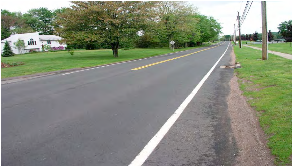
Figure 33 - Visible Image of Figure 32, 2 Years Later– no visible distress.
