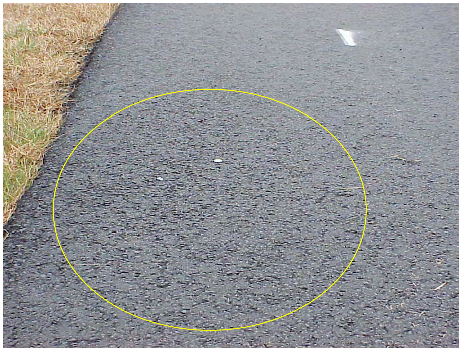
10% RAP, Silo, 1.5" Lift Thickness – Open Texture in Compacted Mat Corresponding to Cold Spot
