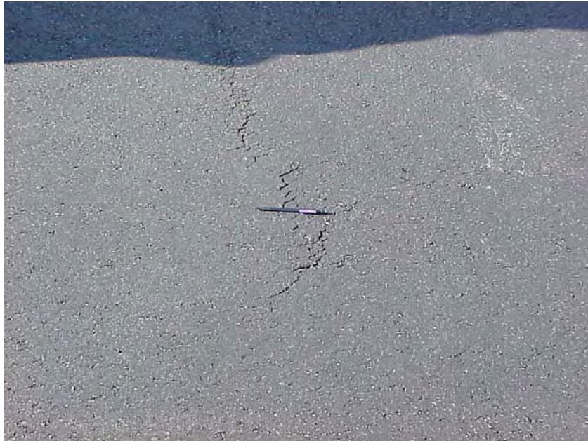
2.0-inch Virgin, No Silo – Cold Rolling Cracks
