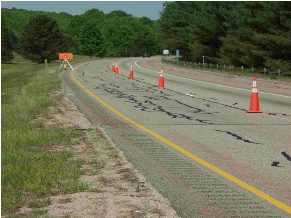
IMAGE #6 - SURFACE CONDITION IN SECTION WB 5, WESTBOUND MILEPOINT 29, (JUNE 2003)
