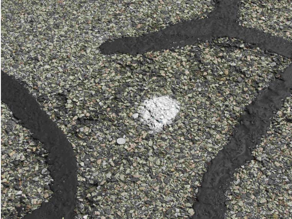
IMAGE #7 - SECTION WB 5, CLOSE-UP OF DETERIORATED SECTION WITH CRACKING AND RAVELING
