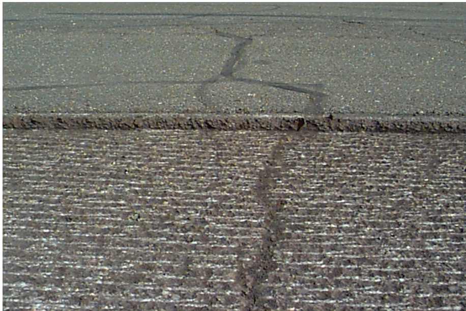
IMAGE #5 CRACKS EVIDENT THROUGH BOTH SURFACE AND MILLED PAVEMENT (MAY 1997)
