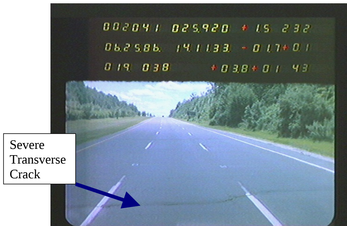
FIGURE 13. ROUTE 2, SECTION WB 6, JUNE 25, 1986. (SEVERE CRACKING THAT EXISTED ONLY AT THE END OF SECTION WB 6)
