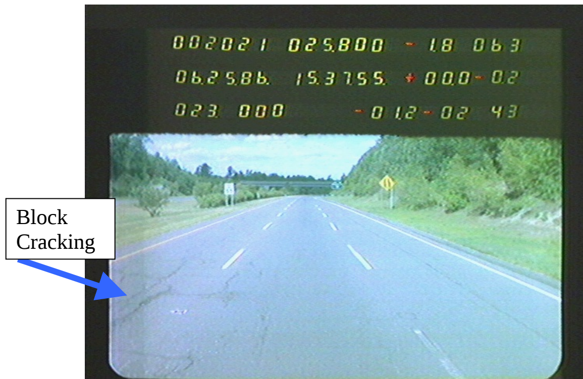
FIGURE 12. ROUTE 2, SECTION EB 1, JUNE 25, 1986 (TYPICAL BLOCK CRACKING PREVALENT THROUGHOUT MOST OF THE PROJECT)
