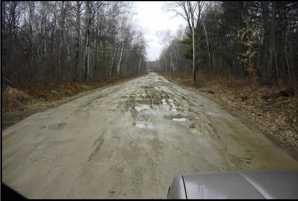
Figure 3.3 Typical road condition of Lakeside Landing Road, Glenburn, Maine in April, 2003.
