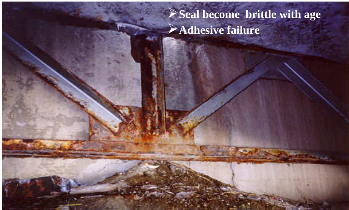
Figure 4. Compression seal leakage.
