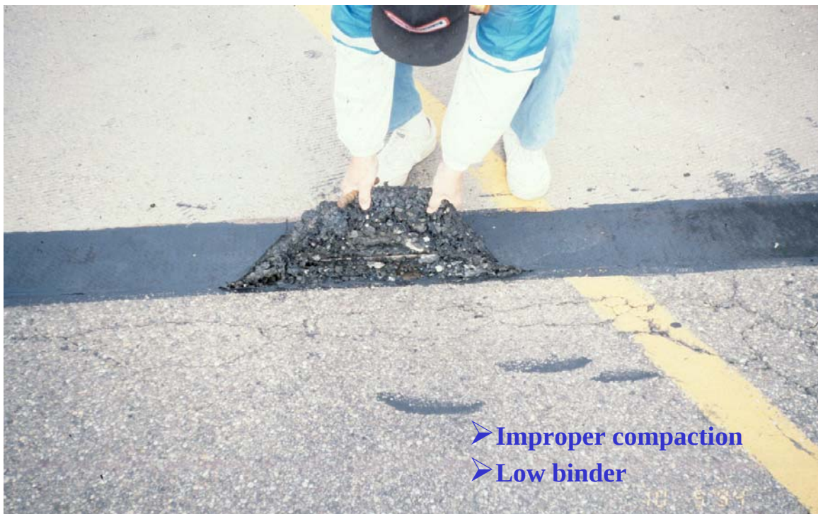
Figure 7. Section of failed joint.
