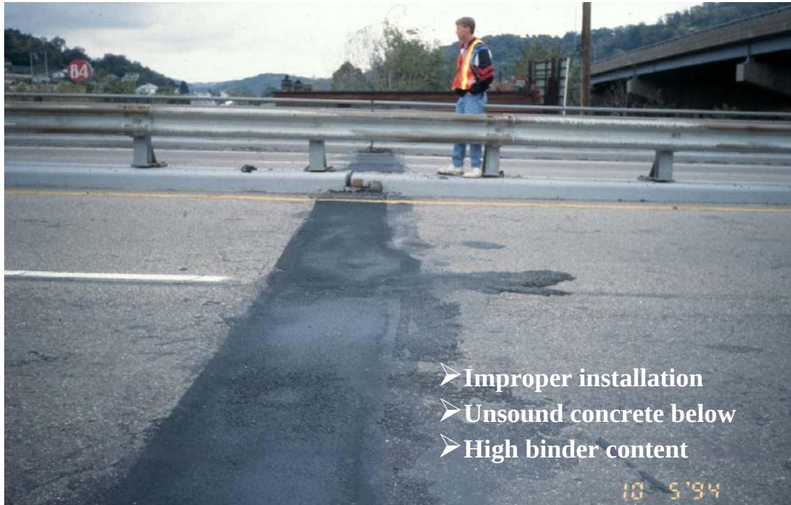
Figure 6. Material flowing on to adjacent pavements.
