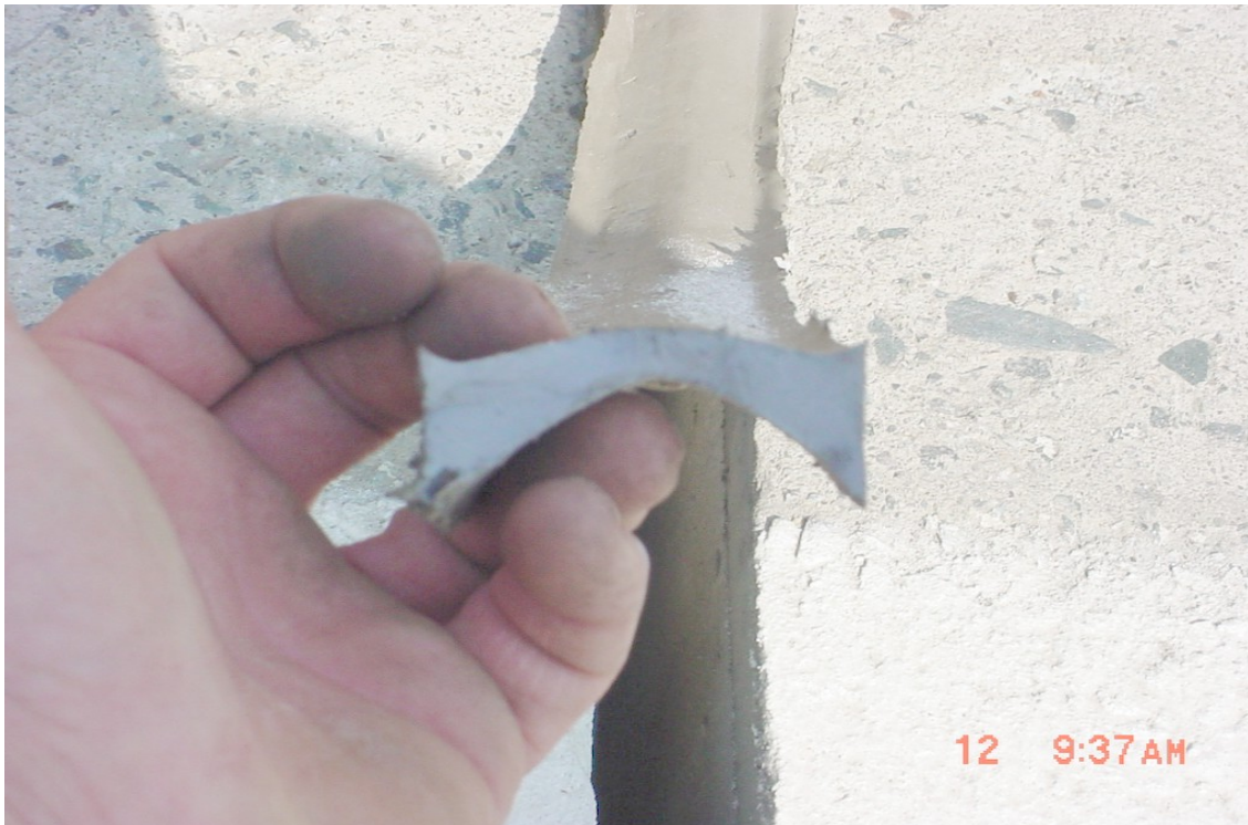
Figure 9. Debonding of silicone sealant.
