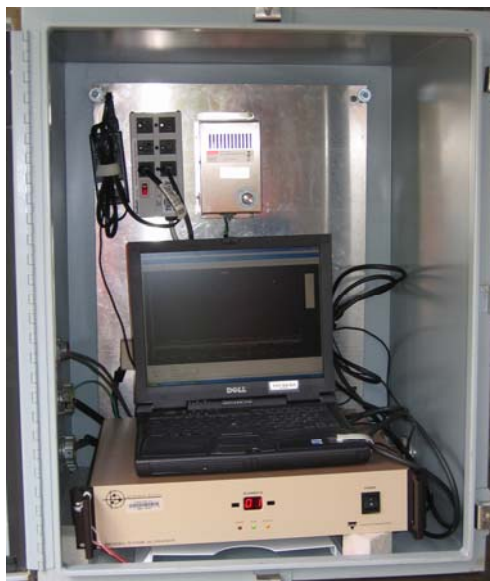
Figure 20 – Monitoring Cabinet for Steel Multi-Girder Bridge
