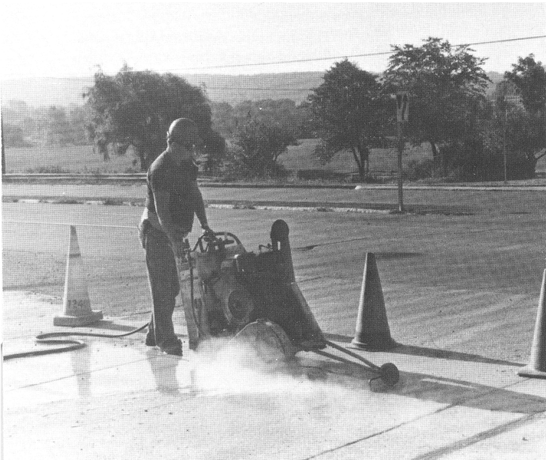
The process of sawing the slot for installation of encapsulated signal wire is improved by using an 18-hp saw rather than a 9.2-hp saw, and by "wet sawing," which reduces hazards to workers and the public due to dust and debris.
