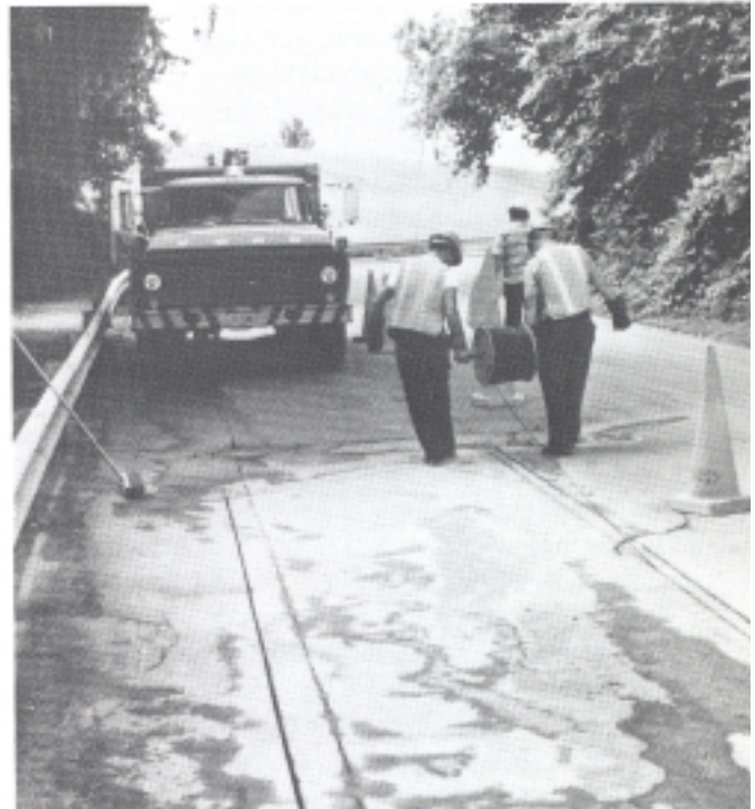
Installation of encased signal wire is as simple as using single-jacketed wire; however, life expectancy of the loop is significantly increased.
