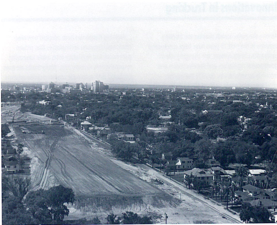
Interstate highway construction in 1963: interchange linking I-75 and I-4 in Tampa, Florida.
