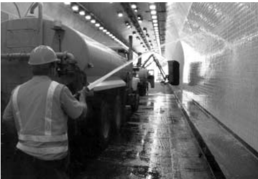
Nevada DOT worker hoses down the tile walls inside the Carlin Tunnels after rotary brushes scrub off grime.
