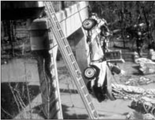
FIGURE 1 Failure of a bridge pier as a result of channel migration led to collapse of bridge over the Hatchie River, Tennessee, in 1989.
