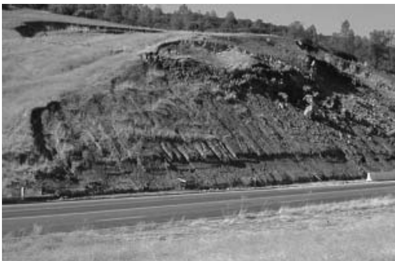
Cut slope failure on Highway 20, Colusa County.
