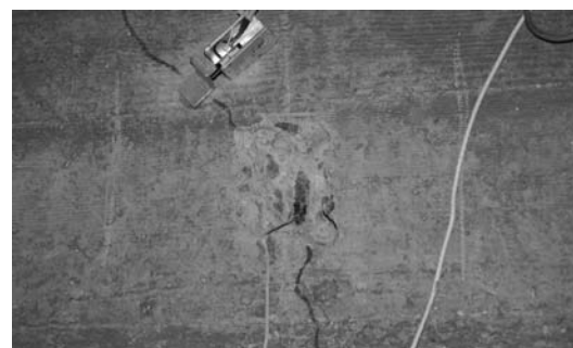
Cracked RCDG bridges were instrumented and monitored.
