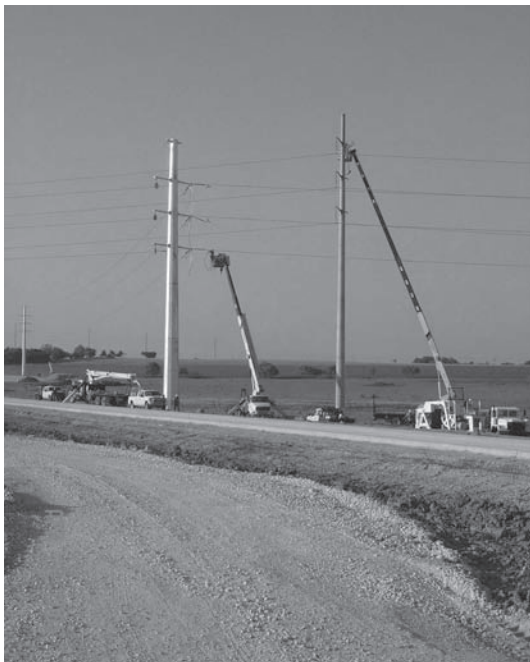
Utility poles are replaced as part of Texas DOT's accelerated State Highway 130 project.
