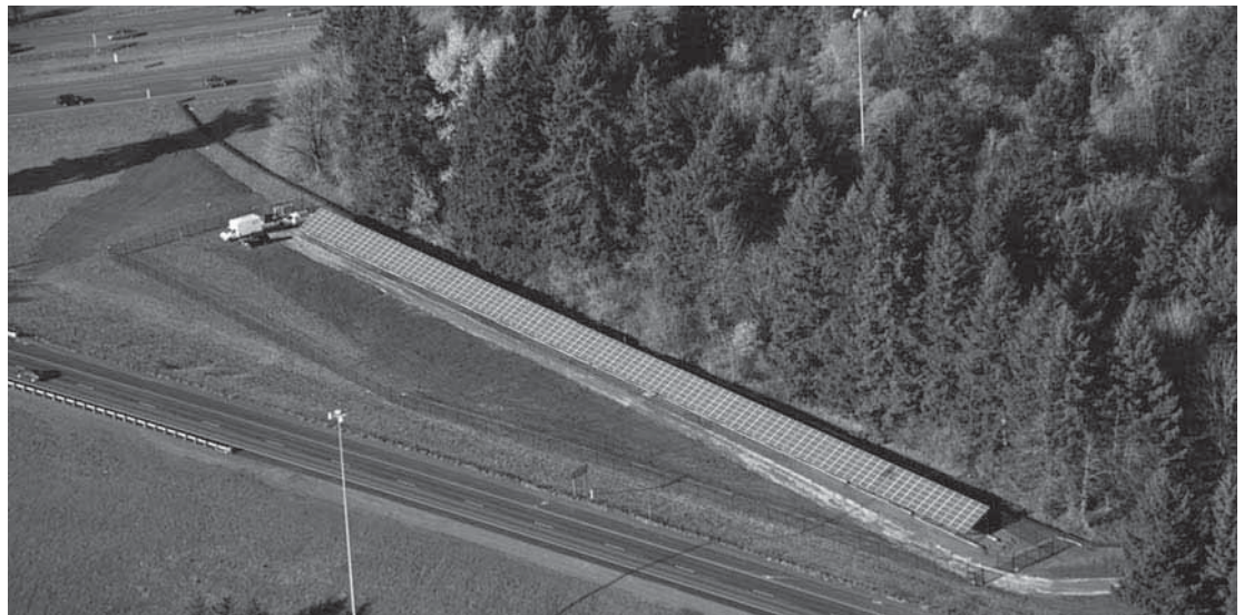
A ground-mounted array of 564 solar panels at the intersection of Interstates 5 and 205, near Tualatin, Oregon, generates 28 percent of the power required to light the interchange at night and reduces pollution.
