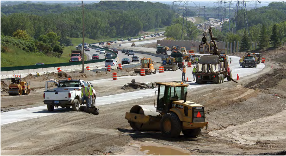
The NCHRP domestic scan team studied Minnesota DOT's right-of-way and utilities relocation procedures for Phase 2 reconstruction on I-494 west of Minneapolis.
