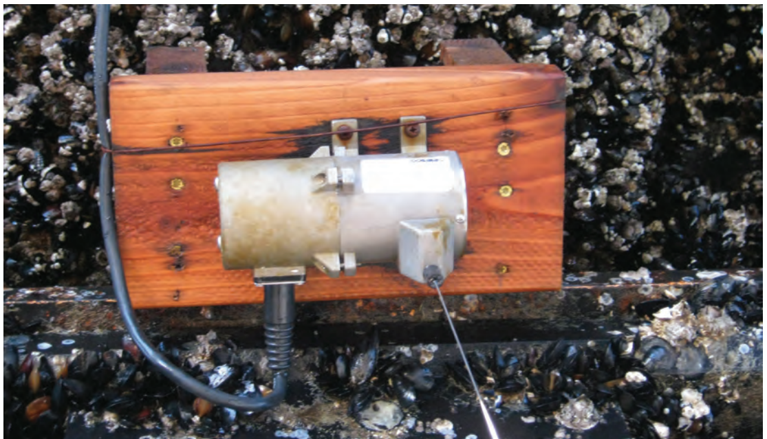
Closeup of linear motion transducer installed in Seattle.
