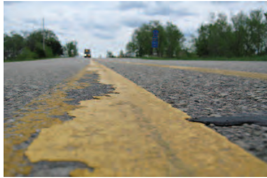
Close-up view of yellow line deterioration.
